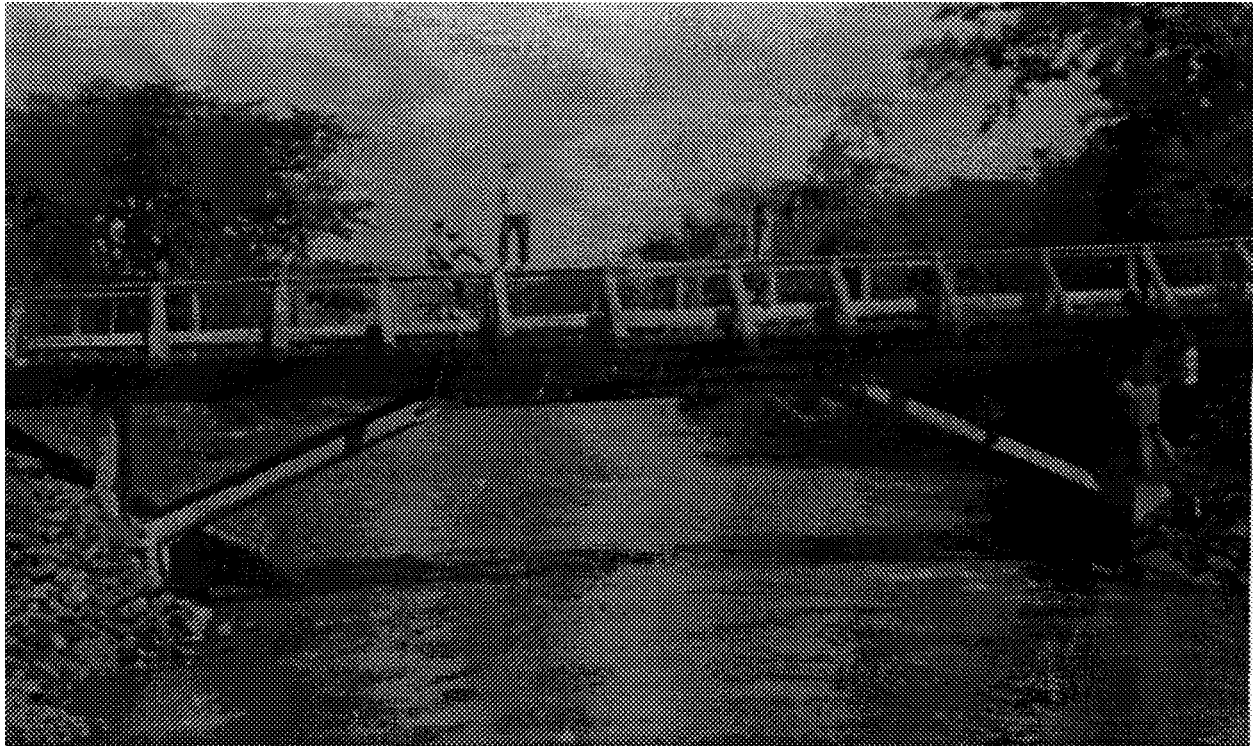
Figure 3. Composite log beam bridge over Ribeirao dos Porcos river. This strut frame bridge is 21 meters long, 15 meters span, consists of four longitudinal composite log beams of eucalyptus specie and was built in 1974.
