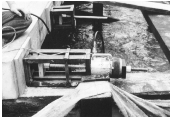
Figure 8—Initial tensioning of the stressing bars was completed with a hollow-core hydraulic cylinder and pump at each successive bar, beginning at one end of the bridge.
