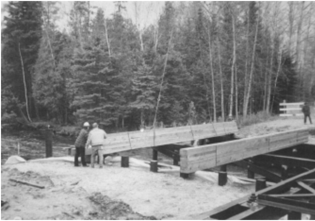
Figure 6—Small crane used to place the strapped lamination bundles onto the abutments.
