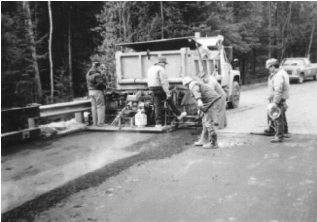
Figure 10—Asphalt pavement wearing surface was applied to the deck approximately 4 weeks after installation.
