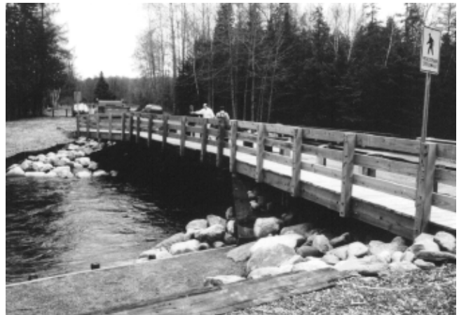
Figure 9—Completed sidewalk structure attached to the superstructure on the downstream side of the bridge.
