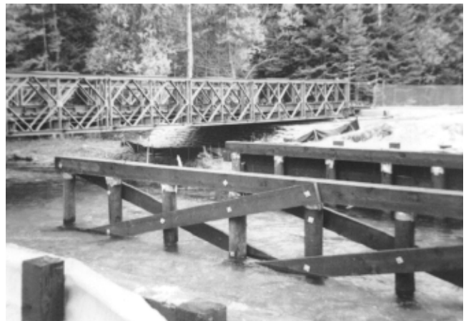
Figure 5—This temporary (Bailey-type) bridge allowed uninterrupted traffic flow across the bridge during the construction of the Graves Crossing bridge.
