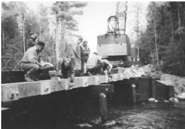
Figure 14—Antrim County personnel collecting load cell readings with a portable strain indicator shortly after the initial tensioning of the stressing bars.
