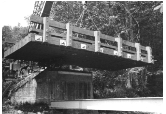
Figure 4—Lifting the prefabricated bridge deck into place with a small crane. Lifting attachments were placed through the deck at several butt joint locations.
