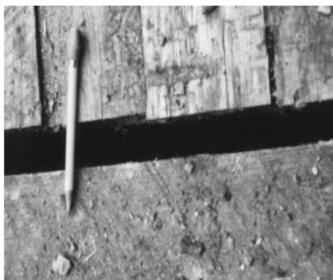
Figure 14—Gap between the bridge end and the substructure backwall at the Tumbling Rock Run bridge.
