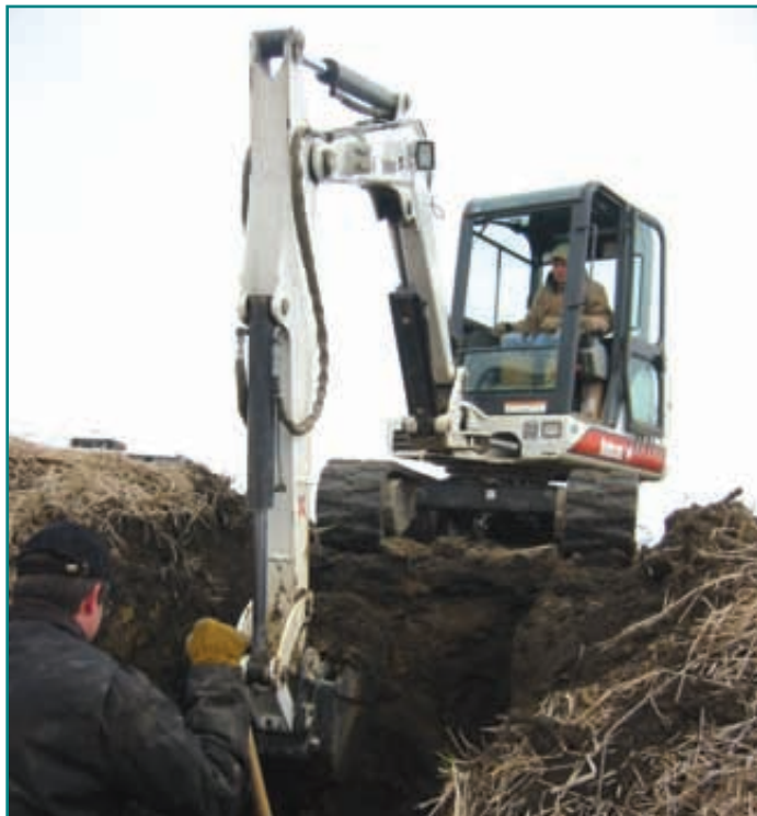
The cost of drainage water management includes installation, as well as purchase and management of the structure.
