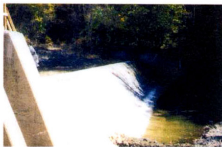
Before removal, the Old Berkshire Mill Dam obstructed the flow of the Housatonic River in Dalton, MA.
