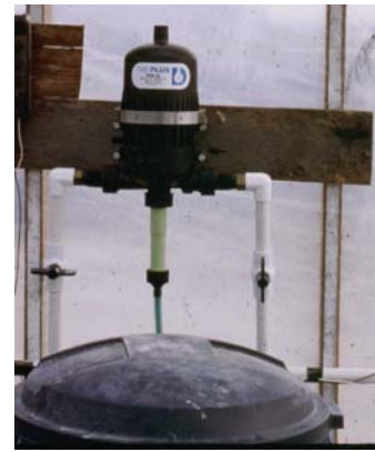
Figure 2 A pump type fertilizer injector used to add concentrated fertilizer to the irrigation water.
