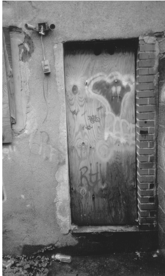
Figure 4: Vandalized Philadelphia Property
