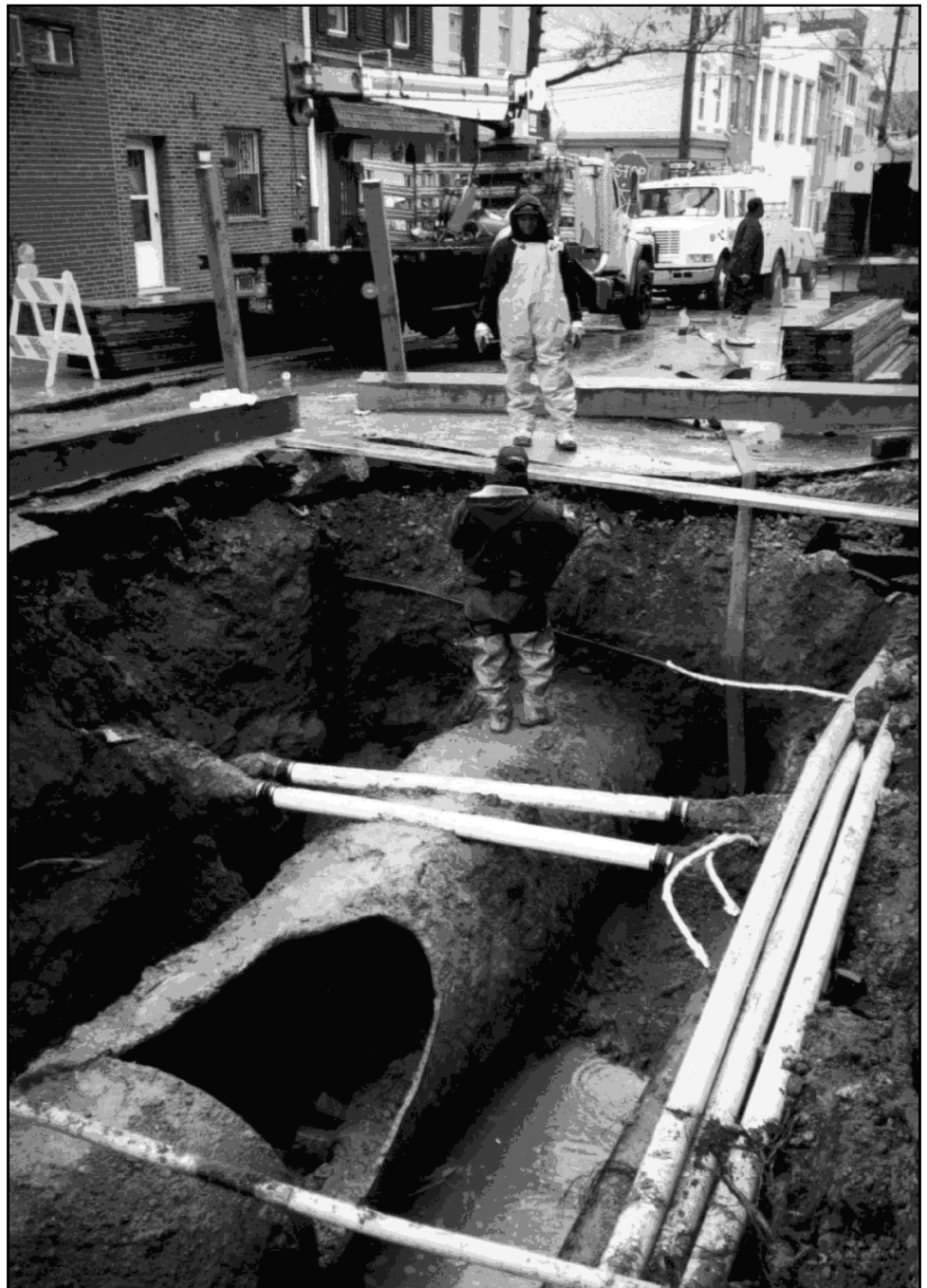
Figure 1: Decaying Drinking Water Pipeline in Philadelphia
