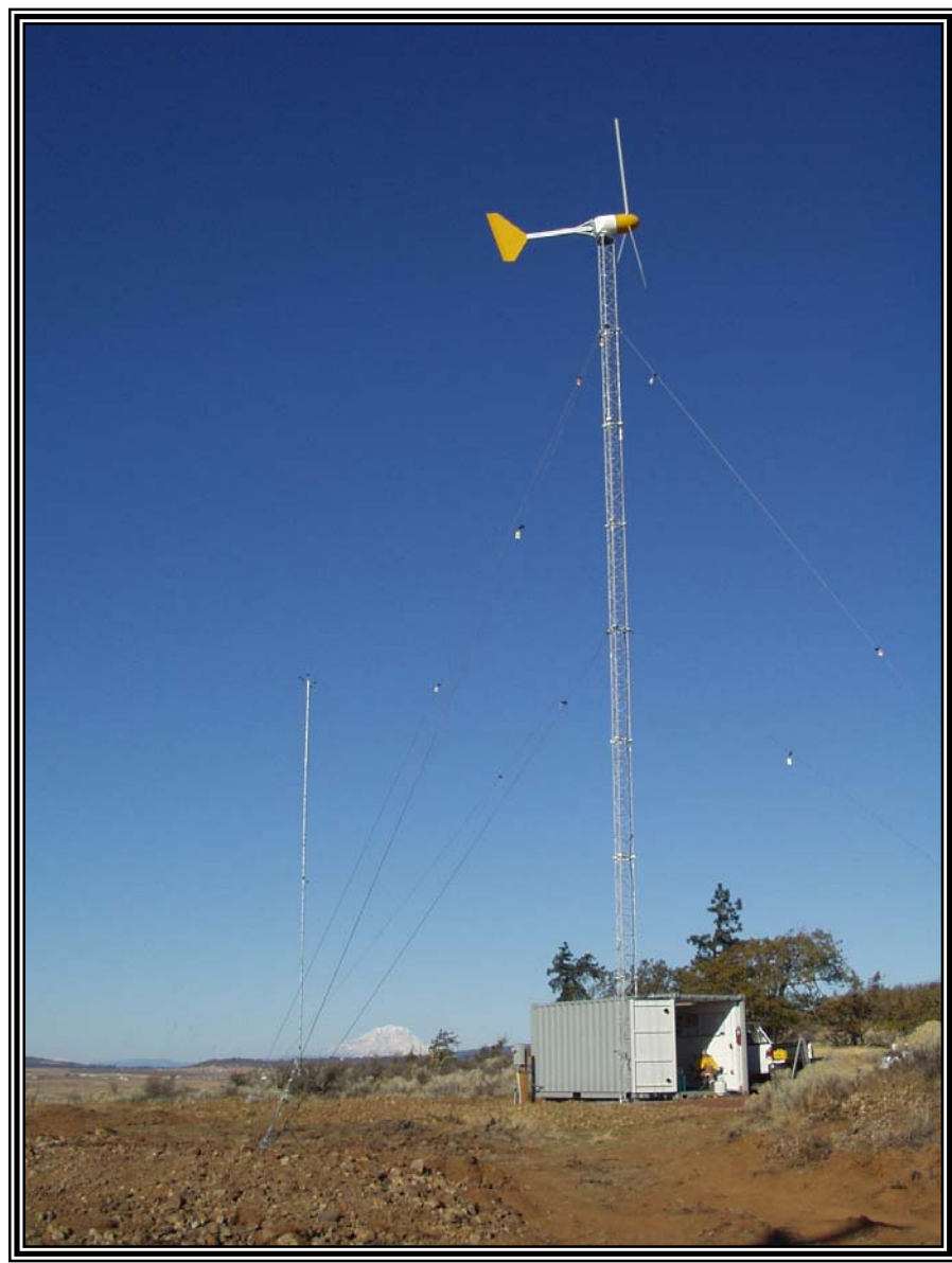
Tower type/height: 24m standard guyed. Commission date October 31, 2003. Host site: Ed Kennell.
