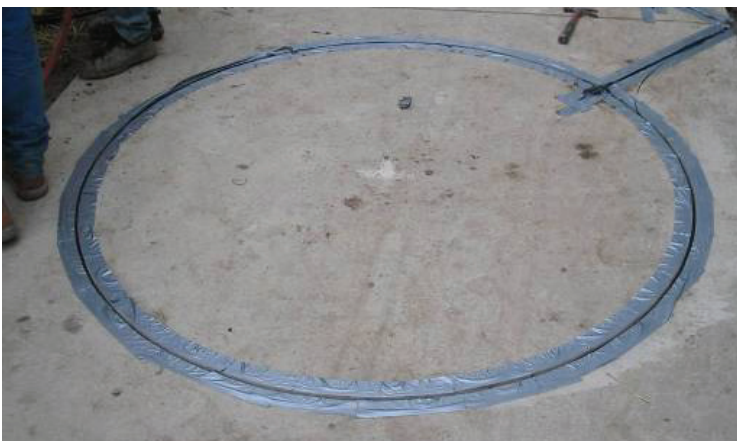
Figure 5-49. Tape placed around both sides of sawcut to prevent sealant from adhering to concrete.
