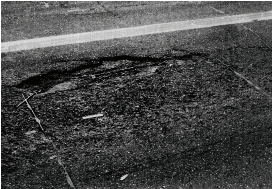
Figure 6-1. Pavement failure near an inductive-loop installation.
