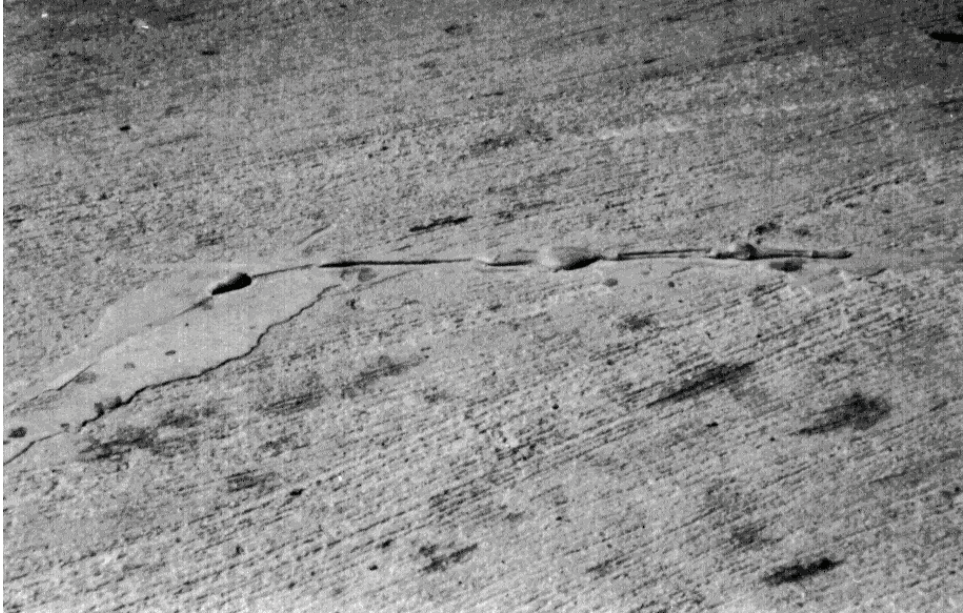
Figure 5-28. Poor sealant application.
