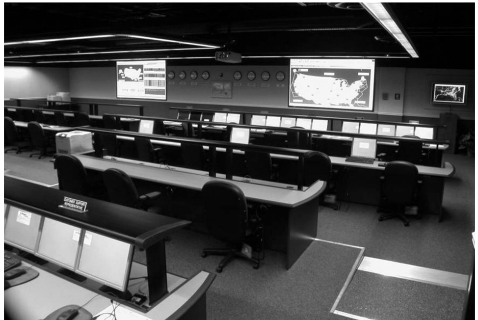
Figure 17: FTI Primary Network Operations Control Center
