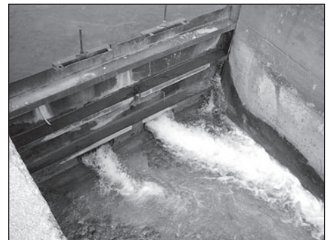
Leaking Check Gate
