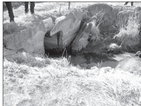
Crumbling Irrigation Structure
