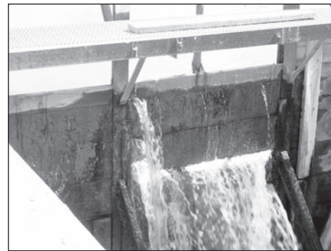
Leaking Check Gate
