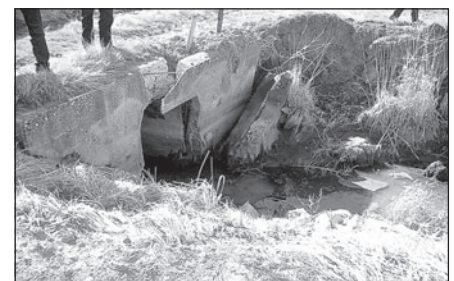
Crumbling Concrete Structure
