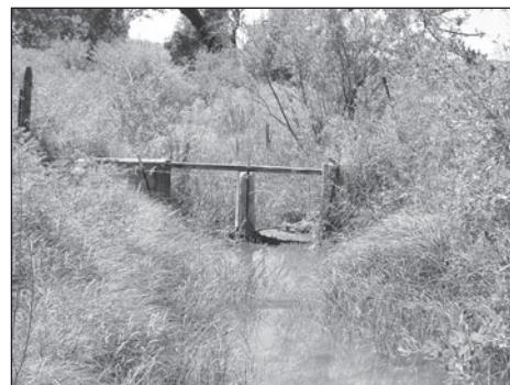
Overgrown Vegetation Around Dilapidated Irrigation Check Structure
