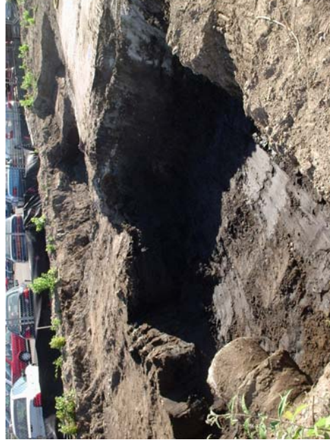
4. Excavation, looking northeast from southwest corner. Note areas of deeper excavation to 5 feet. Note barrier wall on east side of excavation.
