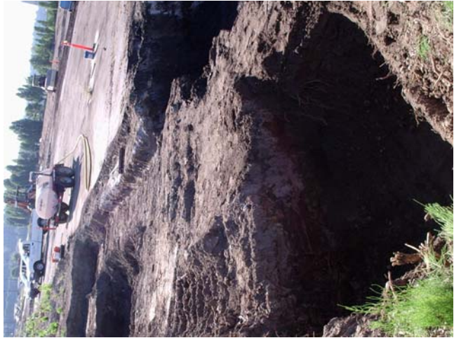
5. 7/21/06 – Excavation looking southeast from northwest corner. Note barrier wall on east side of excavation.
