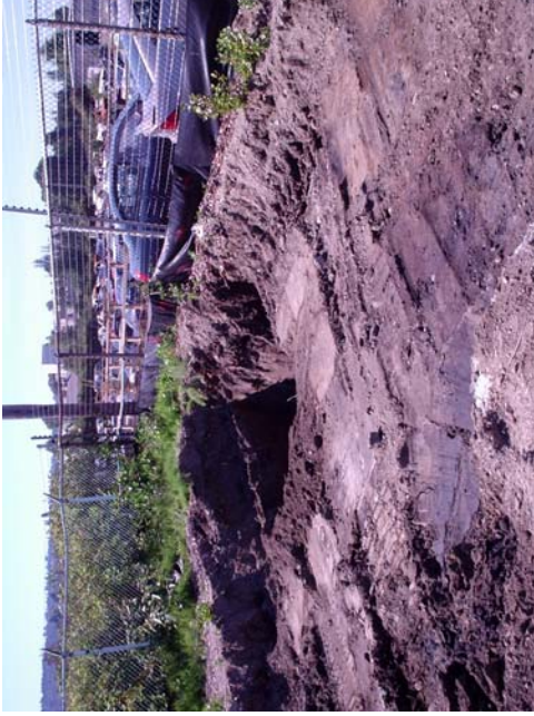
3. Northwest corner of NWC excavation, looking northwest, showing deeper excavation to 5 feet.
