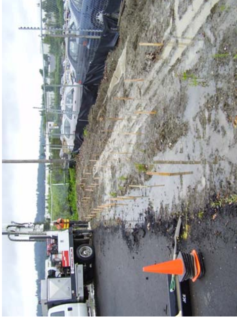
1. 6/2/06 – Northwest Corner (NWC) prior to investigation, looking west; note 35 staked boring locations.
