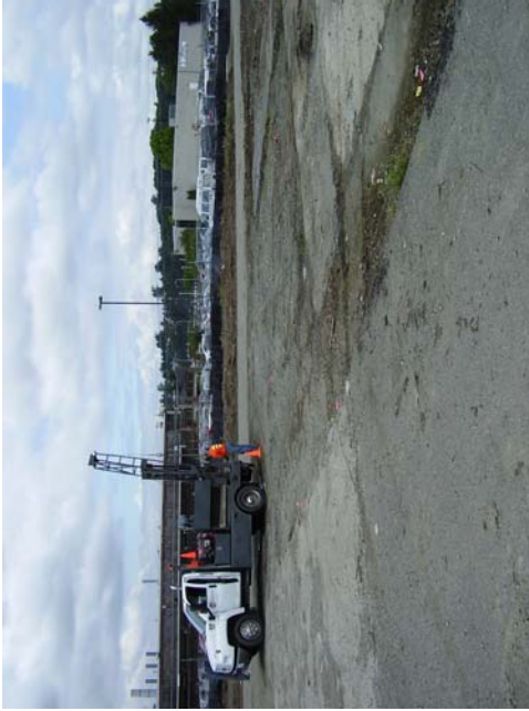
6/9/06 Characterization sampling in Sulfuric Acid Area, looking northeast. Note concrete compressor pad in right foreground.
