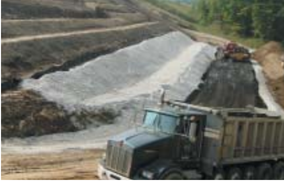
Figure 9. Foundry sand delivery (sand supplied by Kurtz Bros., Inc., construction by Trumbull Corp.)
