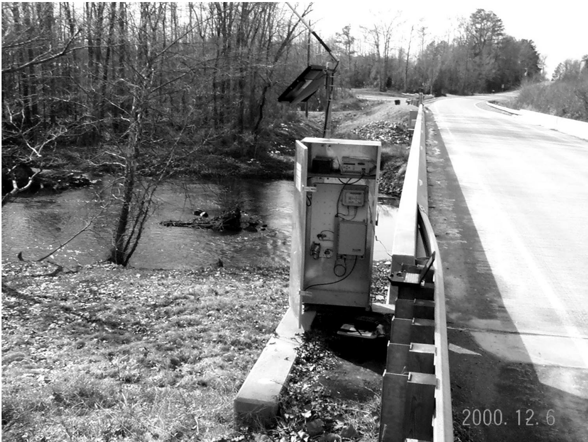
Gaging station at Swift Creek at Hillardston, North Carolina.
