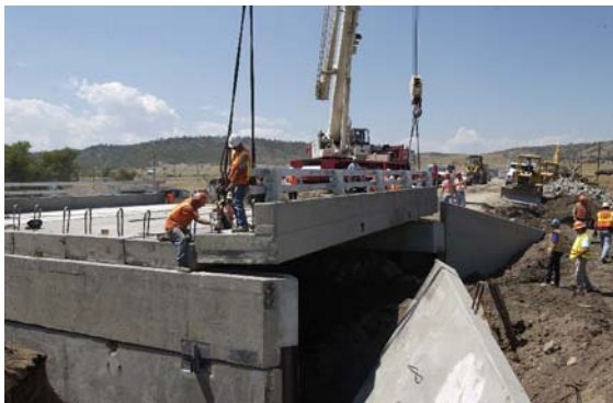
The outside girders were precast with the curb in place and the bridge rail was attached beforehand.
