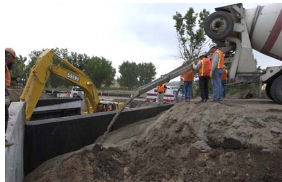
After both abutments were placed, the backface was lined with geofabric and flowfilled.
