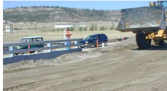
After the girders were post-tensioned together, grouted, and welded to the abutment, aggregate base course (ABC) was placed and compacted.
