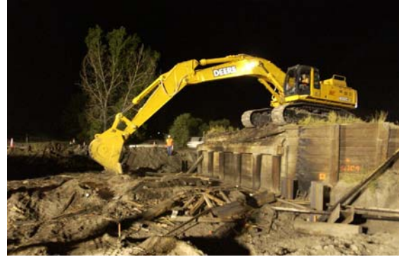
Existing timber pile piers are broken off, abutments and wingwalls are torn out.
