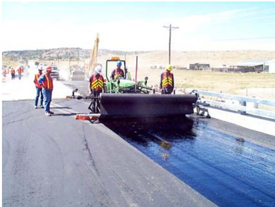
The bottom layer of hot bituminous pavement (HBP) was placed on the ABC, followed by geotextile with a heavy tack coat for waterproofing and abutment reinforcement.
