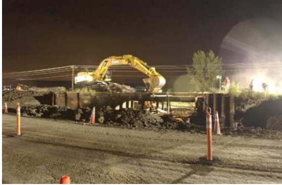
At about 7:30 PM, Friday, demolition began. The old bridge was rapidly ripped apart and moved out of the way.
