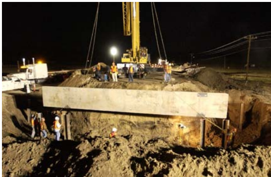
The first precast member, the west "hide wall" is delivered shortly after midnight.
