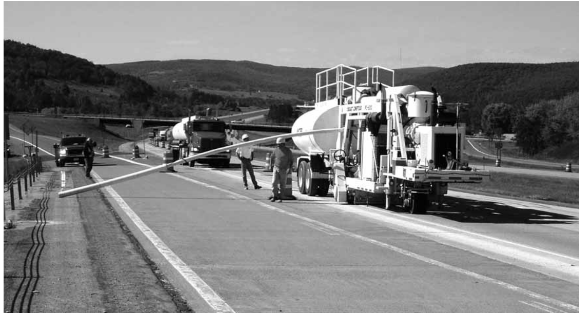
Pavement preservation treatments must be carefully selected and must be applied before the pavement sustains structural damage.
