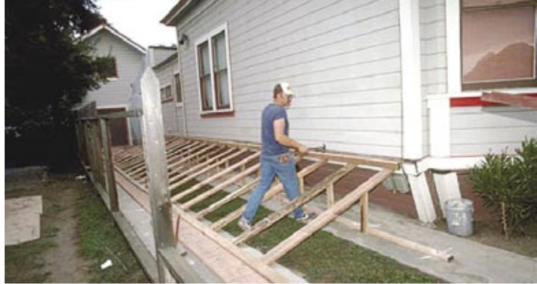
Houses without adequate connections to foundations can easily shift during even moderate earthquake shaking, causing extensive damage. Pipes and wires may be broken by a slight cripple-wall shift, resulting in fires, water damage or other problems. Much damage of this type can be avoided by using inexpensive bracing techniques, such as those recommended in the seismic design provisions of building codes.
