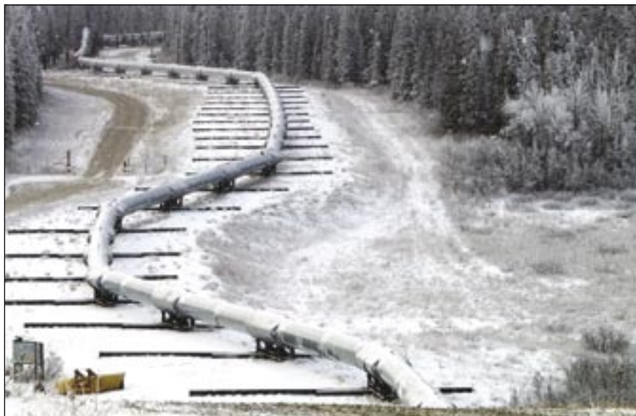
Designed to withstand a magnitude-8 earthquake with up to 20 feet of movement, the Trans-Alaska Pipeline is supported by rails on which it can slide freely during an earthquake.
