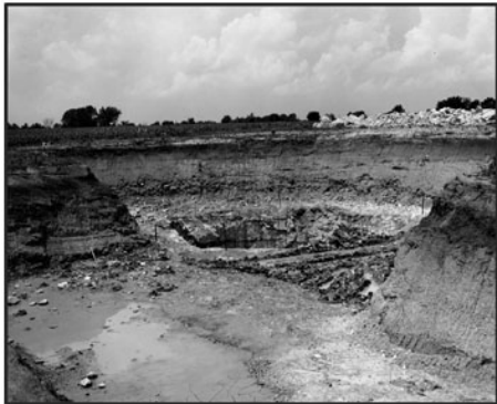
Historic photograph of Minuteman II construction. Courtesy of Whiteman Air Force Base, Oscar I Museum, 1962.
