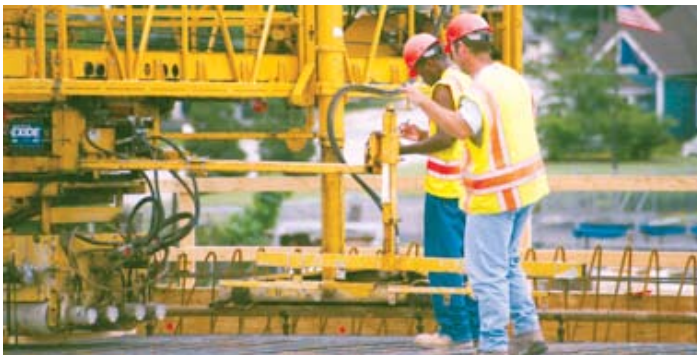
Working on the I-70 Hyper Fix Project (I-65 / I-70) in Indianapolis. Photo courtesy of Heather Miller.
