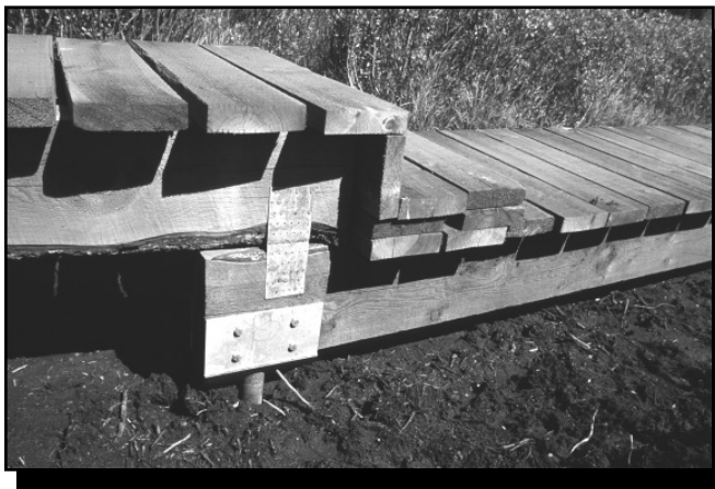
Figure 38—A helical pile was used for this boardwalk. Stringers are attached directly to the beam saddle, helping to keep the boardwalk close to the ground.
