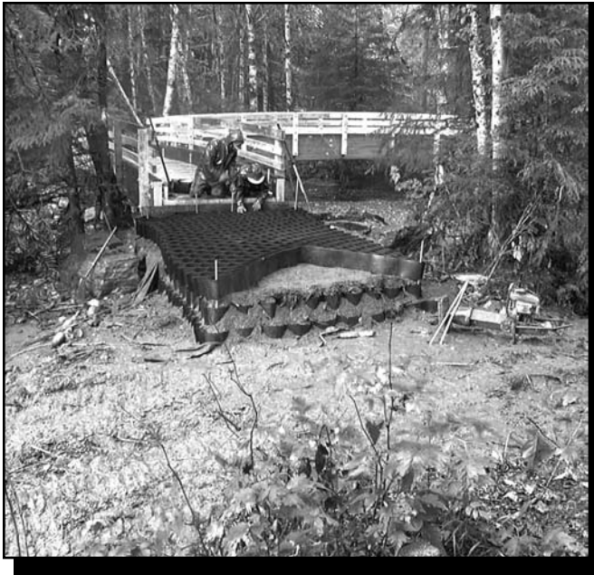
Figure 72—Geocell being laid in courses for a bridge approach. When the approach is completed, the geocell will not be visible.
