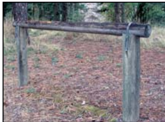
Figure 10–42—Because stock chew on wood hitch rails, the crossmembers eventually weaken.
