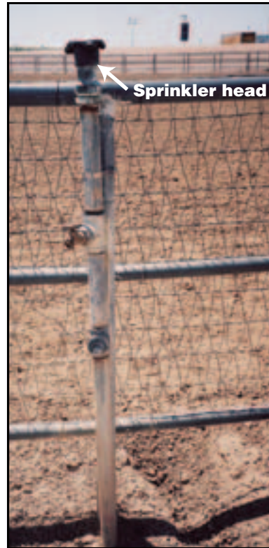
Figure 10–65—Sprinkler heads can be placed on the top fence rail. Another popular location is at ground level. Regardless of the location, the sprinkler heads should be placed so they are not hazardous to riders or stock.
