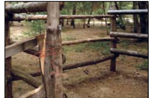
Figure 10–26—Baling twine provides a temporary—and possibly unsafe—field fix for a broken gate. Schedule regular inspection and maintenance for gates and fences in recreation sites.
