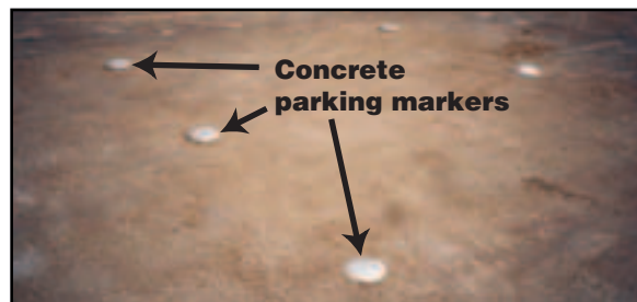
Figure 8–16—Concrete markers are used to delineate unpaved parking spaces in some areas of the country.
