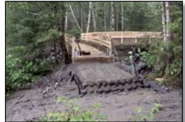
Figure 5-10—Workers have compacted soil into layers of geocell to provide stability at a bridge approach. The top layer will bring the tread level even with the deck level.
