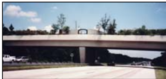
Figure 5-27—The Marjorie Harris Carr Cross Florida Greenway Land Bridge across Interstate Highway 75 south of Ocala allows riders, hikers, and bicyclists to cross six lanes of traffic. The bridge is 52.5 feet wide and 200 feet long.
