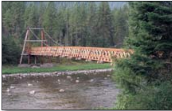
Figure 5-19—This wood suspension bridge is designed for packstock use in a wildland setting. The design would be appropriate for other users in other settings.
