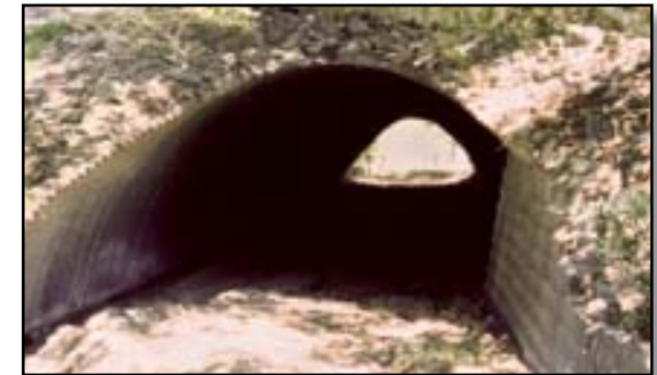
Figure 5–33—Riders need more lateral clearance near the top of underpasses than other users. Provide 12 feet of overhead clearance that is the entire width of the trail. Avoid sloping roofs that force riders to the center of the tread.
