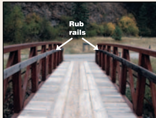
Figure 5-25—Wood rub rails are frequently used on bridges to keep saddles, backpacks, bicycle handlebars, and other equipment from snagging on posts.
