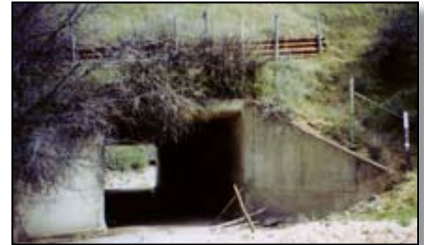
Figure 5–32—When selecting equestrian underpasses, such as this common box culvert, carefully consider overhead and horizontal clearance.
