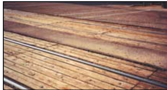
Figure 5–7—Building a horse trail in an active railroad corridor requires extensive negotiation to address safety and liability concerns for trail users and railroad personnel. If trails must cross tracks, the tread should be level and the gaps filled according to railroad requirements. Trails also must approach tracks at a 90-degree angle.
