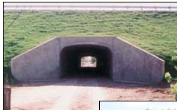
Figure 5-29—Underpasses can have different configurations, such as this one with approach wings. — Courtesy of Bridgetek.
