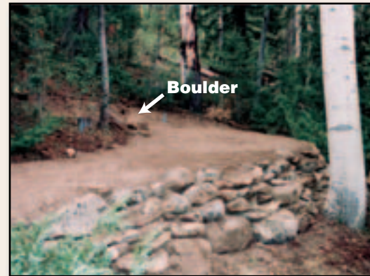
Figure 4–22—This newly reconstructed switchback includes a landing reinforced with a retaining wall. A boulder placed at the inside of the turn prevents shortcutting.
