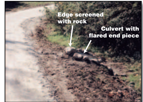
Figure 4-20—This trail culvert has a flared end piece that is partially concealed with rock. It is attractive, durable, conforms to the slope, and improves waterflow. Culverts with flared or covered ends are more horse-friendly than exposed culverts because they look more natural and there is no exposed metal to make noise when a horse steps on it. — Courtesy of Kandee Haertel.
