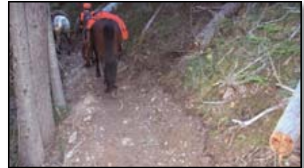
Figure 4-14—When constructing hillside trails in steep terrain, excavated soil is cast downhill.
