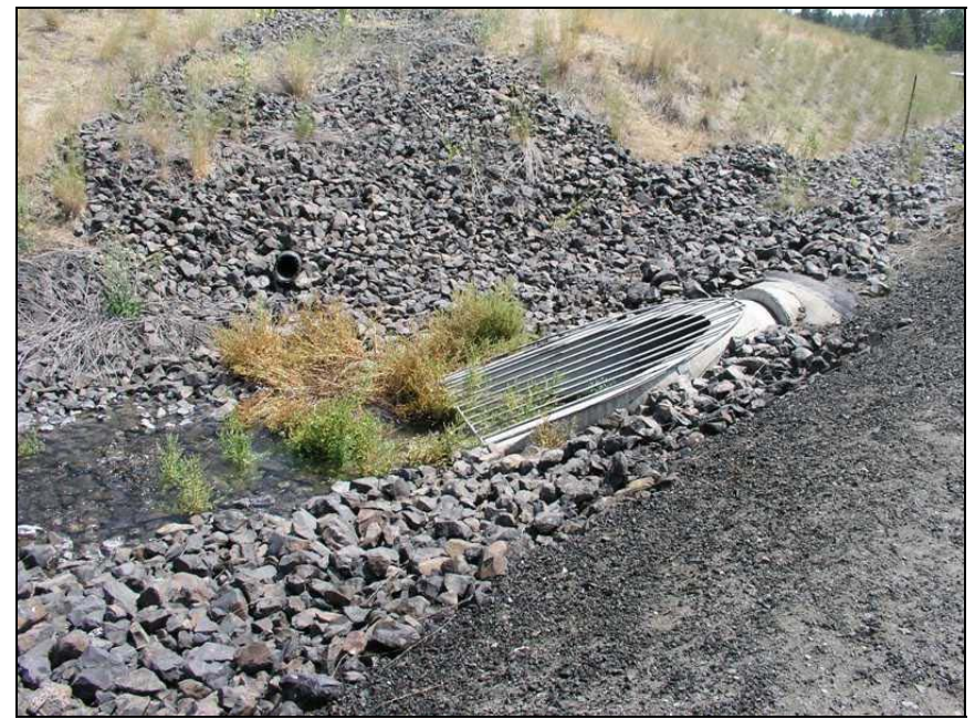
Surface water collection drain on west side of landfill access road
