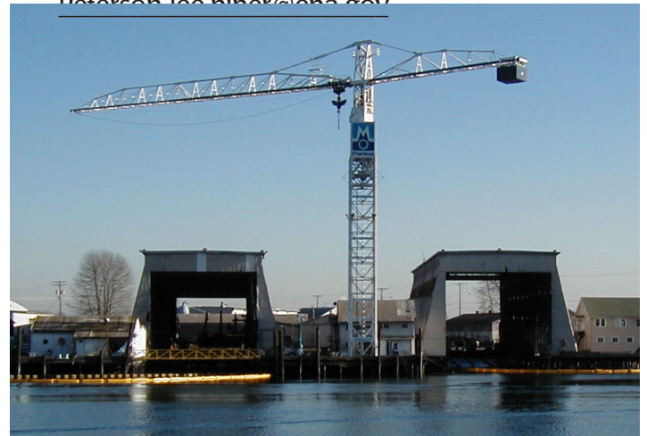
Earlier this year, debris was removed and 3 feet of capping material placed underneath the buildings and docks at Martinac Shipbuilding Corp.
