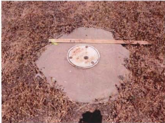
Monitoring well W-7
