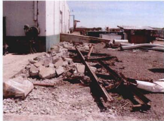
Demolition of old railroad spur looking east towards the southwest corner of Stephens Metal Products warehouse
