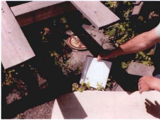
Monitoring well W-13
