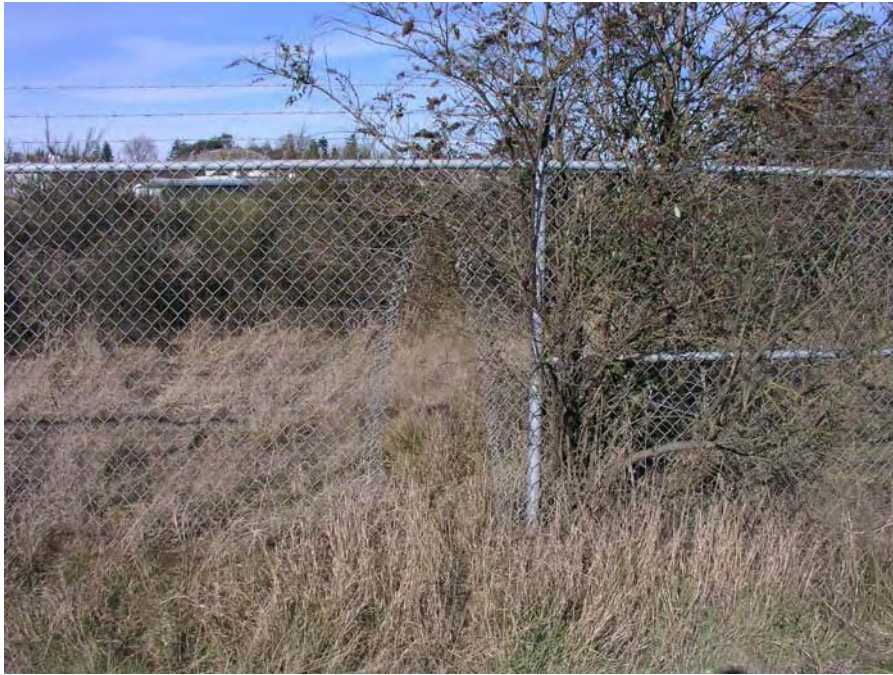
Photo 1. Hole in North Containment Area Fence
