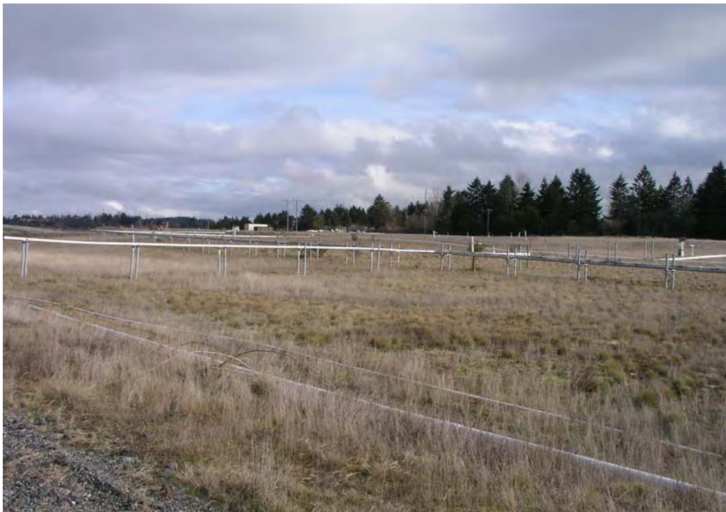
Photo 2: Landfill cap and gas extraction system piping.
