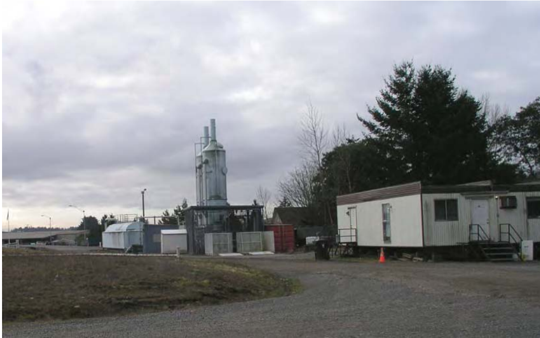
Photo 3: Mothballed ground water treatment facility.
