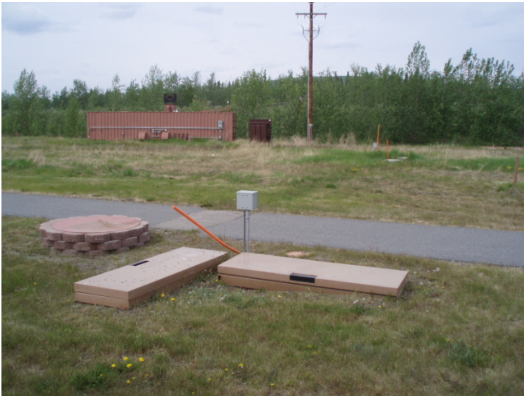
Photograph 23 – Sparge Curtain Treatment System Operable Unit 5
