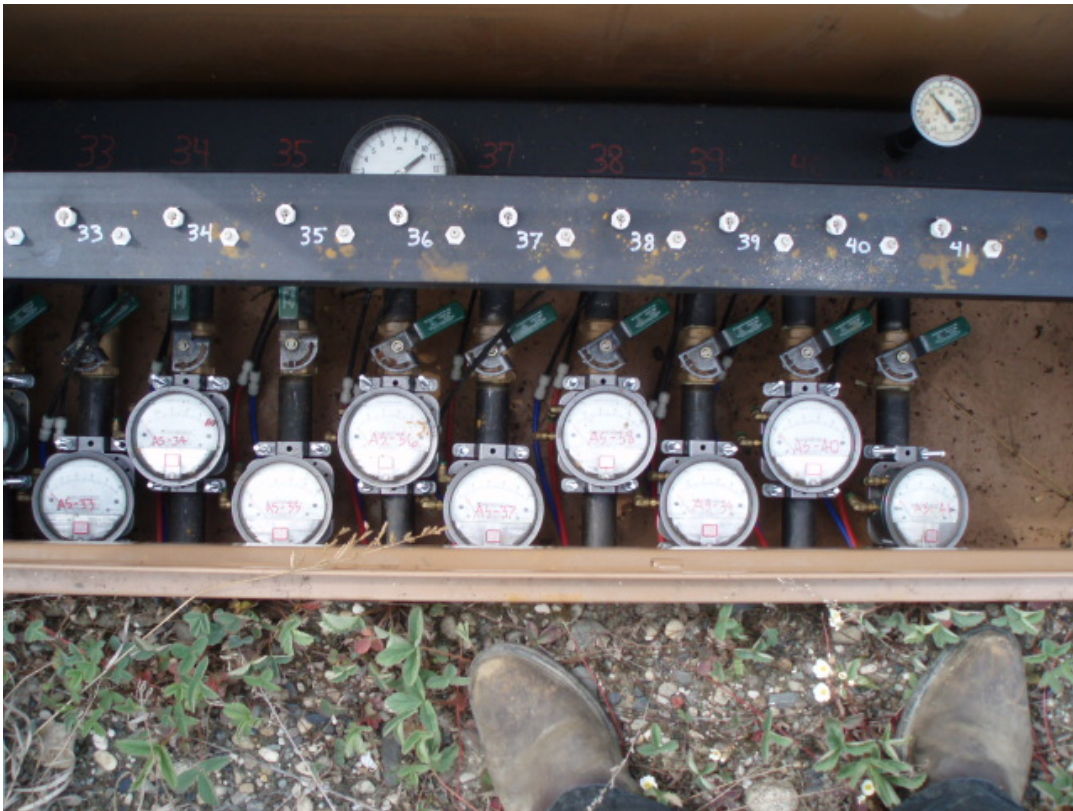
Photograph 27 – Interior of Monitoring Enclosure Operable Unit 5
