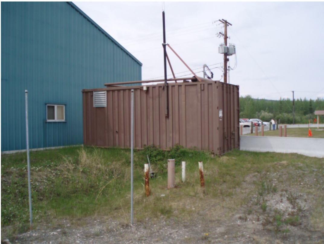
Photograph 28 – Building 1060W Treatment System Operable Unit 5
