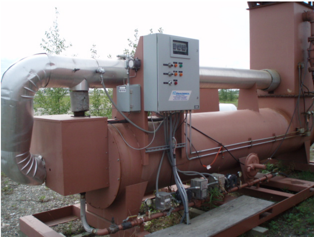
Photograph 26 – Thermal/Catalytic Oxidizer, Source Area Treatment System Operable Unit 5
