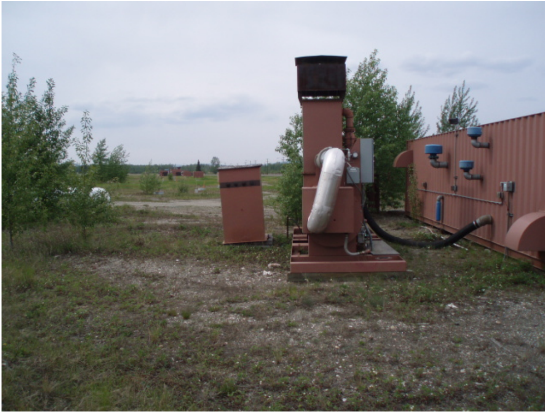
Photograph 25 – Source Area Treatment System (Horizontal Well Treatment System Visible In Background), Operable Unit 5
