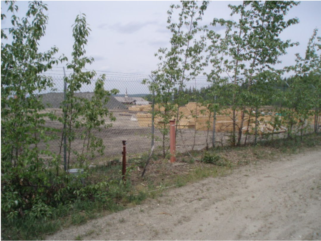
Photograph 15 – Post Fence Line along Thaw Channel Area (New Housing Development Construction in Background), Operable Unit 3
