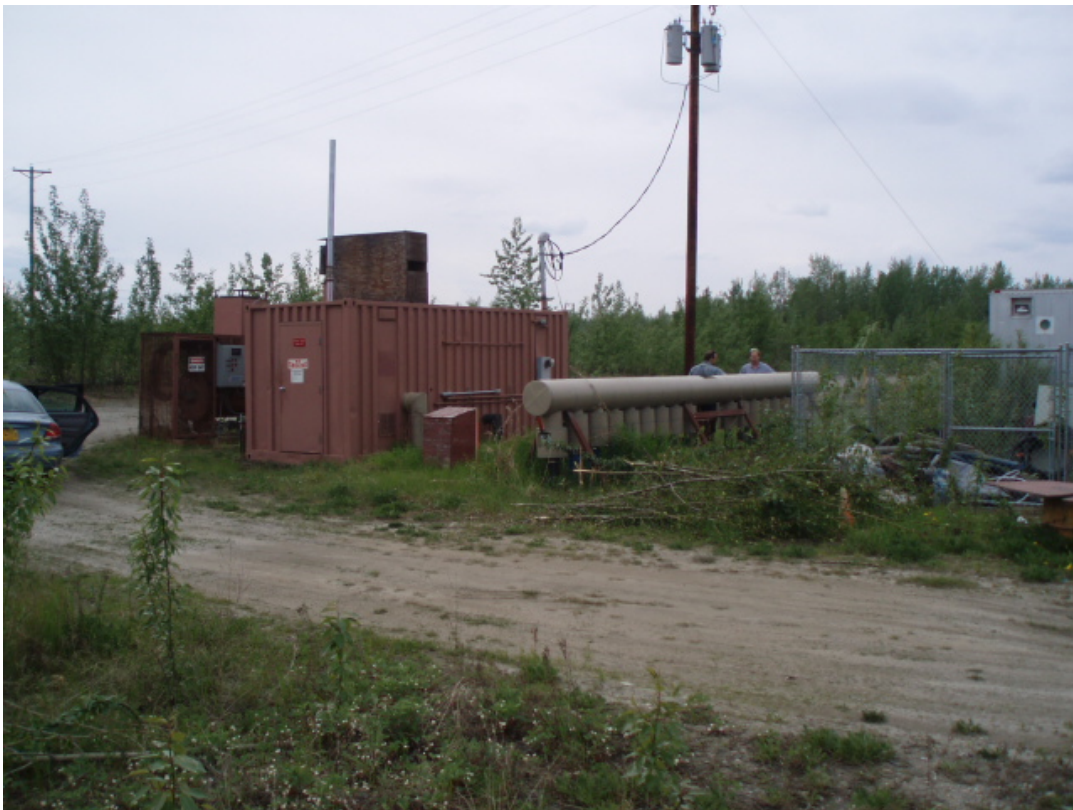
Photograph 18 – Central Header Treatment System Operable Unit 3
