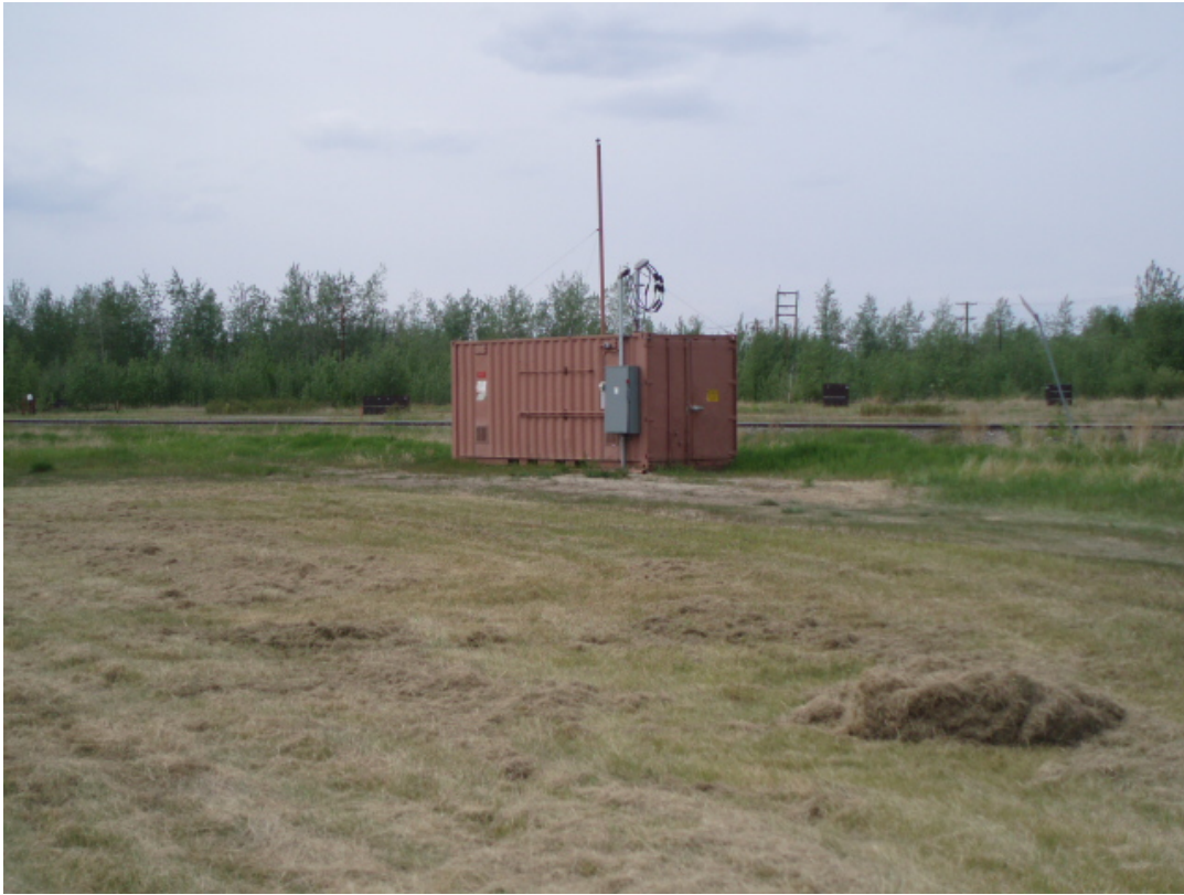
Photograph 17 – Eight Car Header Upgradient Area Treatment System Operable Unit 3
