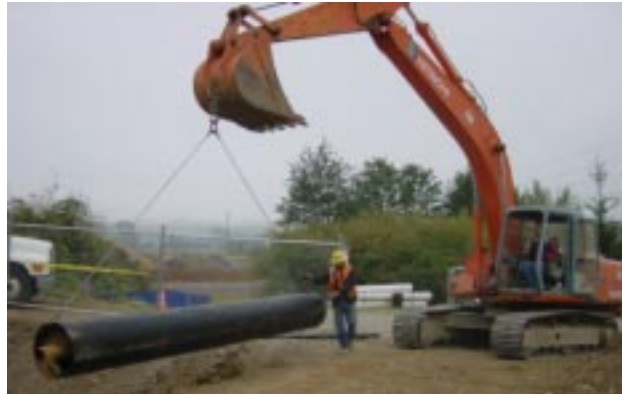
Workers lift a piece of the new water line into place at Hamilton/Labree site.
