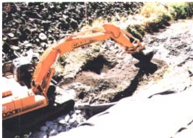
Workers remove PCB-contaminated sediments from Truax Creek at Teledyne Wah Chang site.
