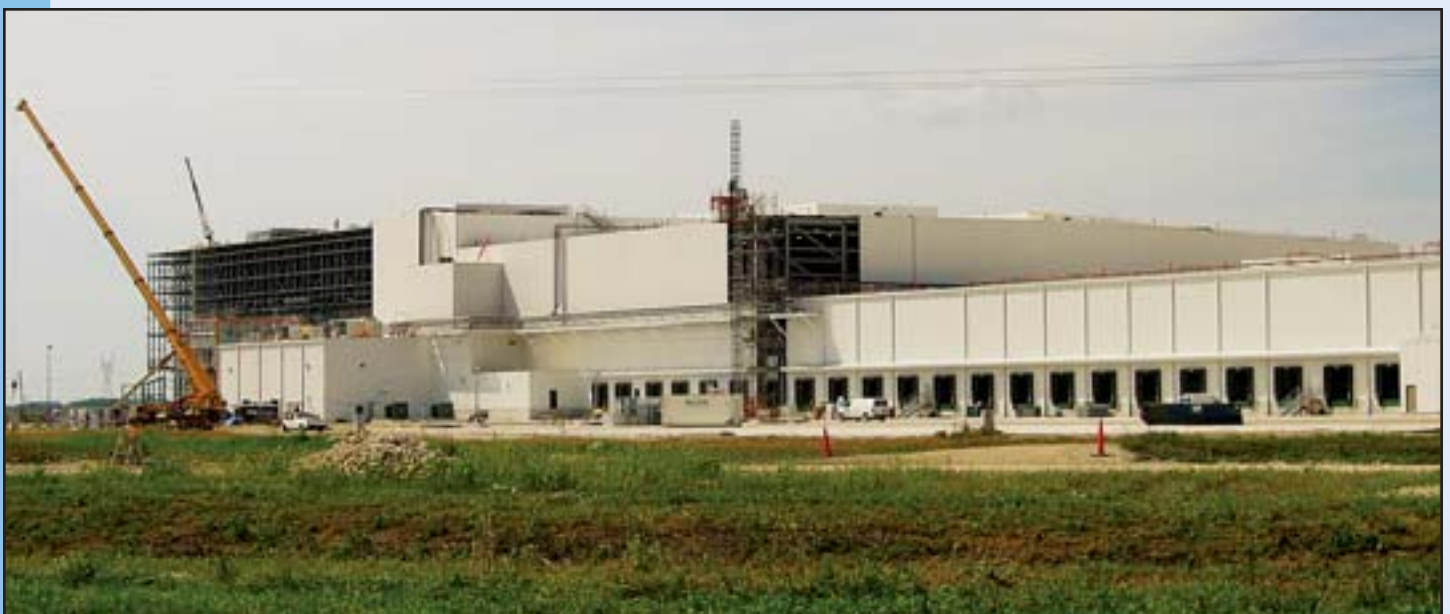
A Wal-Mart distribution center under construction in Sterling, Illinois at the former Sterling Mill site.
