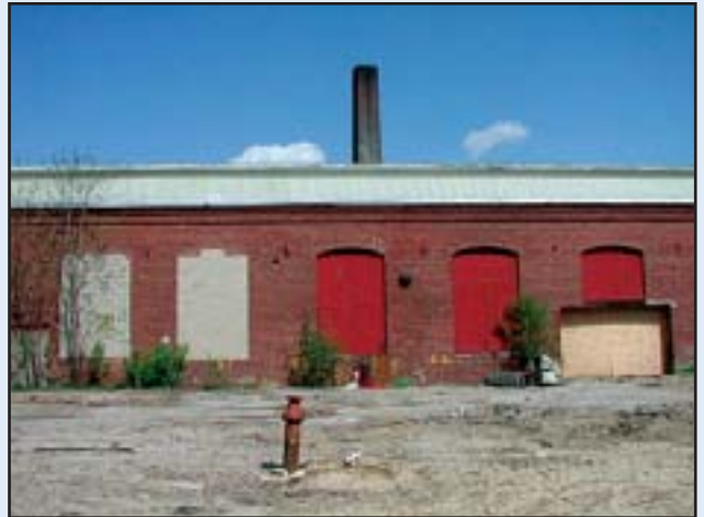
The front view of the Allen Rogers Wood Turning Mill in Laconia, New Hampshire, before redevelopment.
