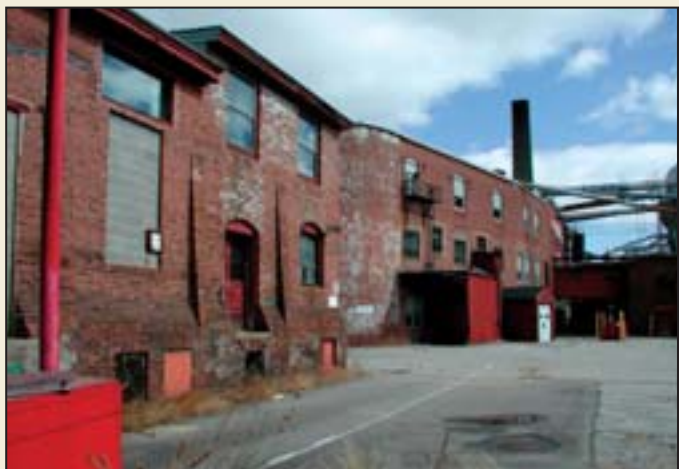
The rear view of the Allen Rogers Wood Turning Mill before redevelopment.
