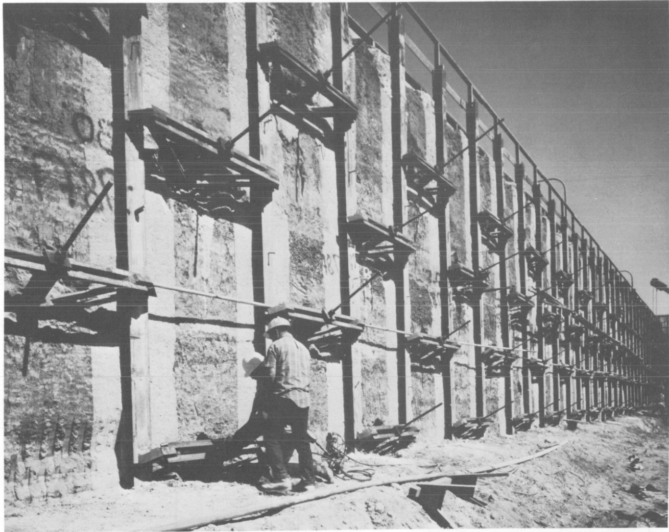
Figure 77. Example of tied-back wall using channel sections as wales. (Courtesy of Hughes Tool Company).
