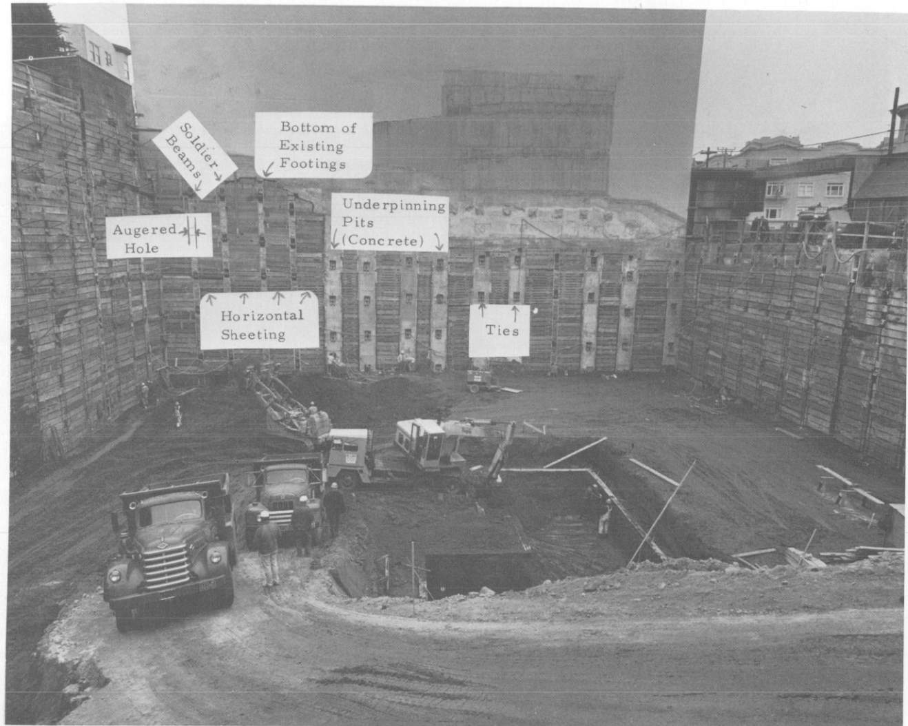
Left side shows augered hole with steel soldier pile and lean concrete backfill. Right side shows pit underpinning and interpit sheeting.
