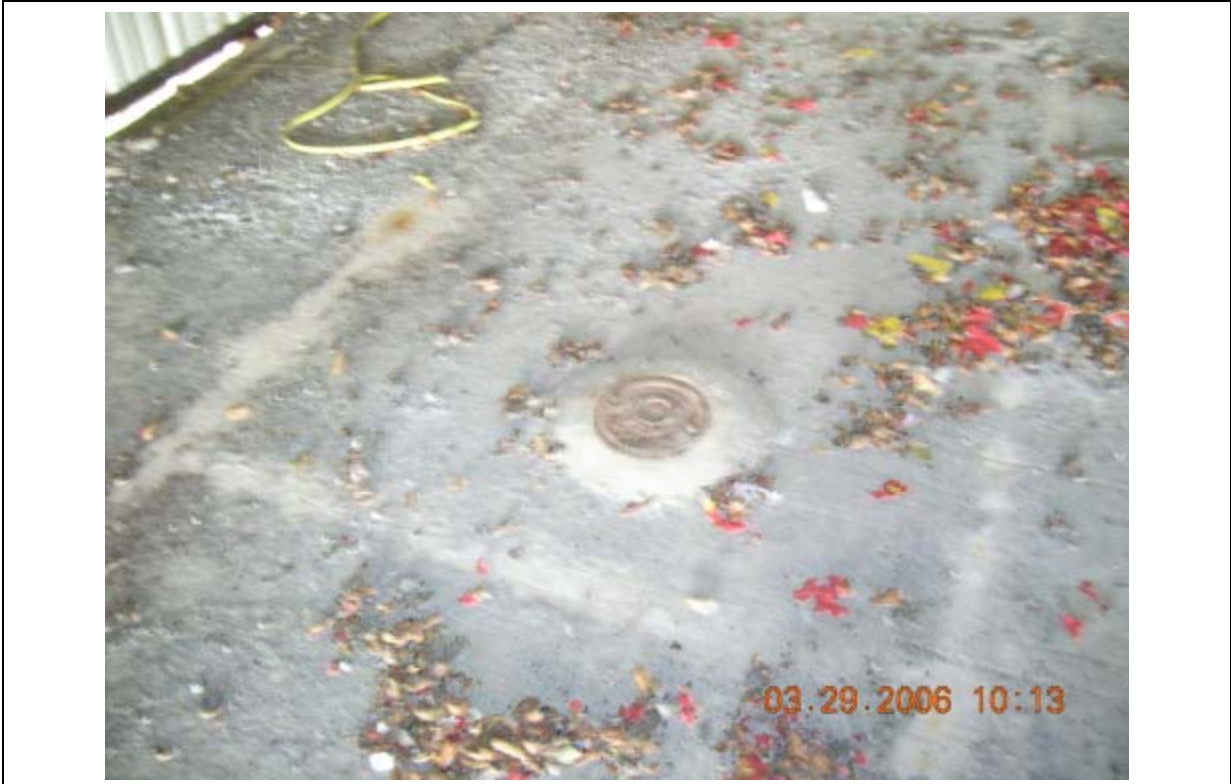
Photo 7: View of monitor well MW-09, located inside Process Building No. 1.
