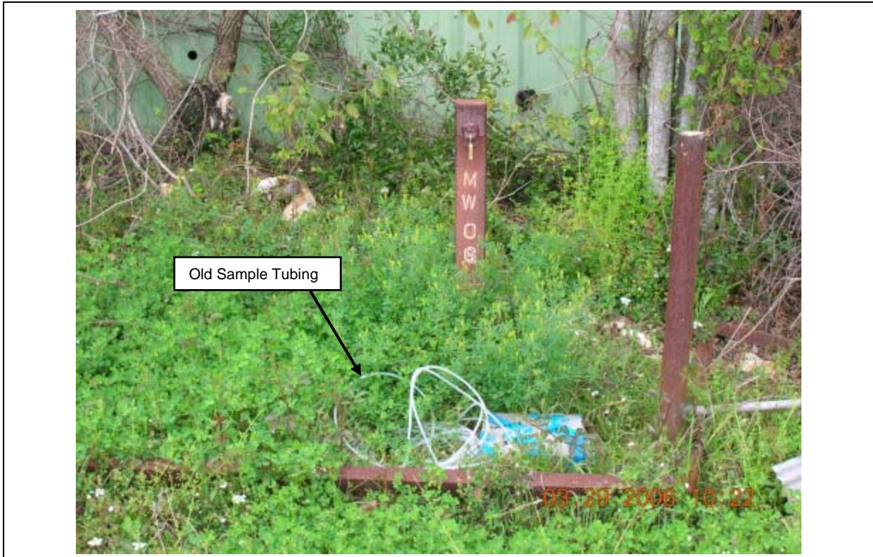
Photo 9: View of monitor well MW-06, located on east side of Process Building No. 1. Old sample tubing is lying on ground next to the well.
