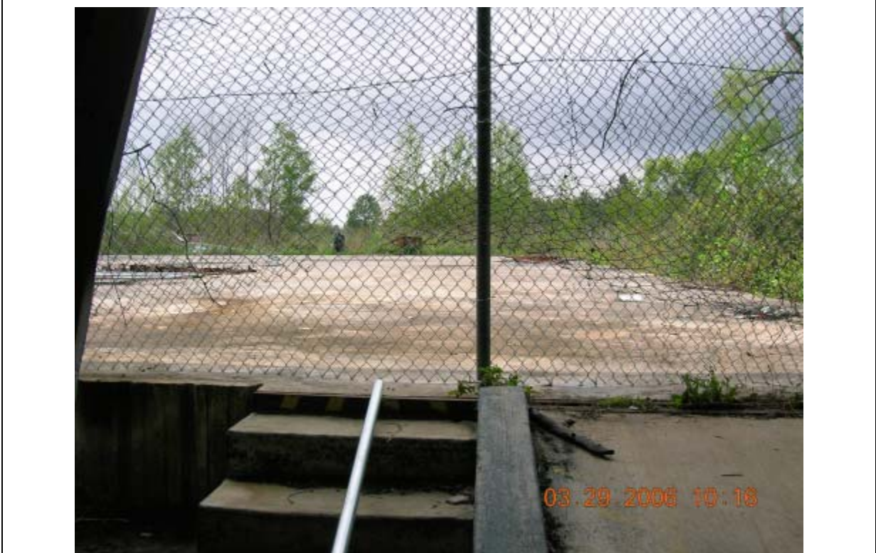
Photo 8: View of fence at doors on south side of Process Building No. 1, facing south. Fence was repaired due to trespassers.
