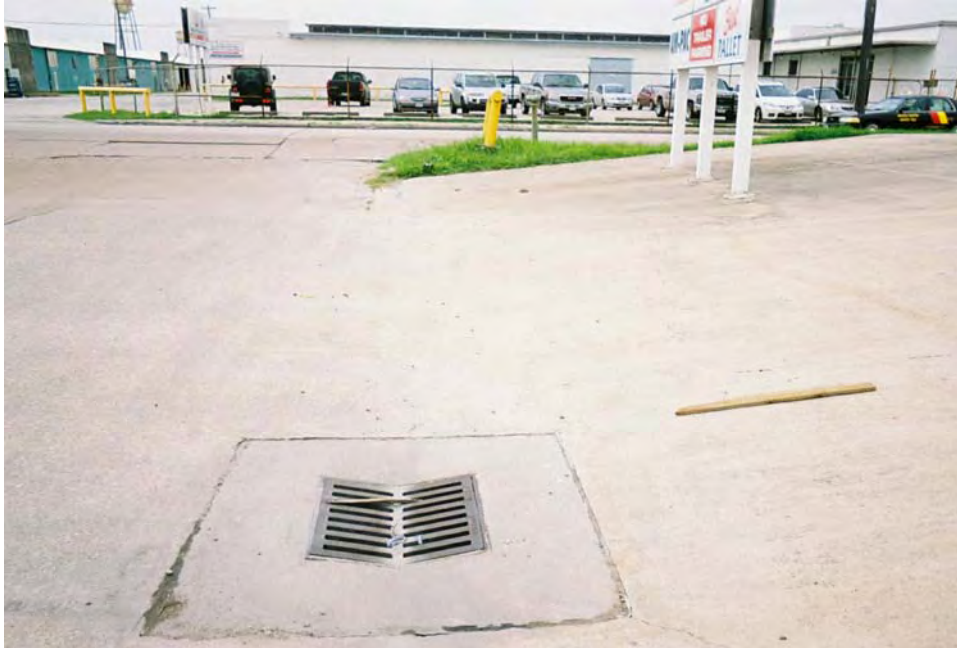
View looking south towards Collingsworth Street showing a storm drain adjacent to the southwest cap
