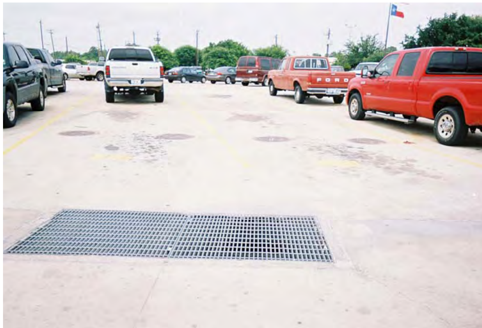
View looking west showing storm drain and detention basin covers in the southeast area
