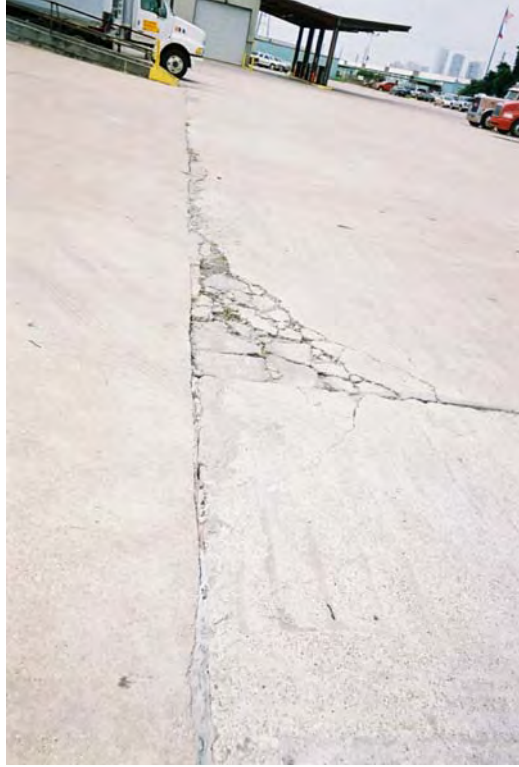
View looking south showing cracked concrete outside the southeast cap area
