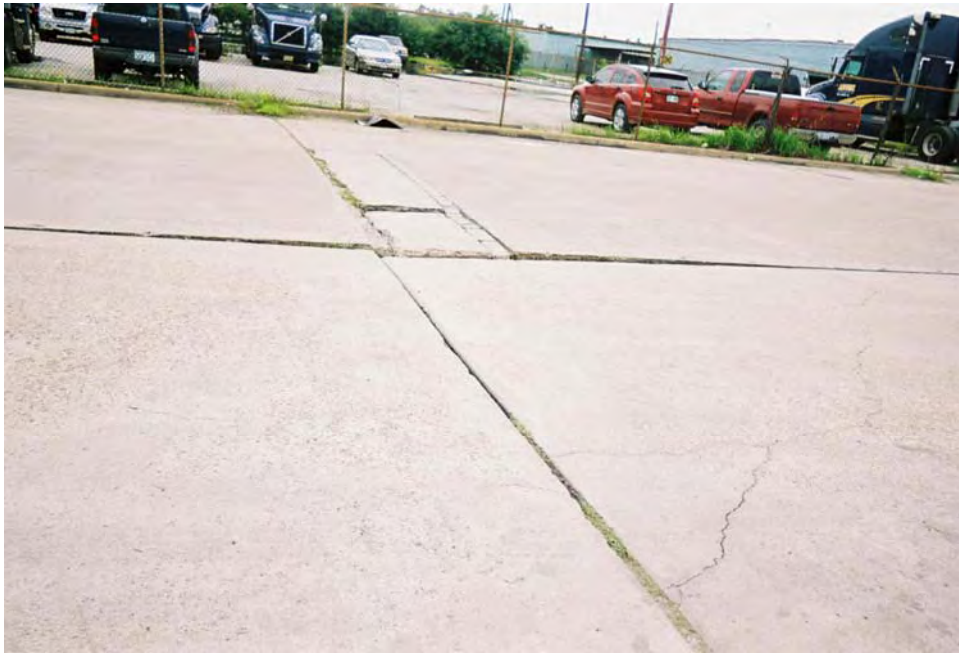
View looking east showing driveway in the southwest area which is offset along the joints
