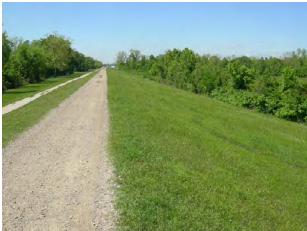
Photo 24: View along Mississippi River levee, facing northwest. Site is located to the right behind trees.
