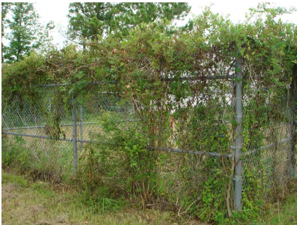
Photograph No. 11 Site: Highlands Acid Pit Superfund Site Description: Vegetative overgrowth on cluster fencing; Date: June 20, 2007 maintenance activities indicated it had been recently cut at the base
