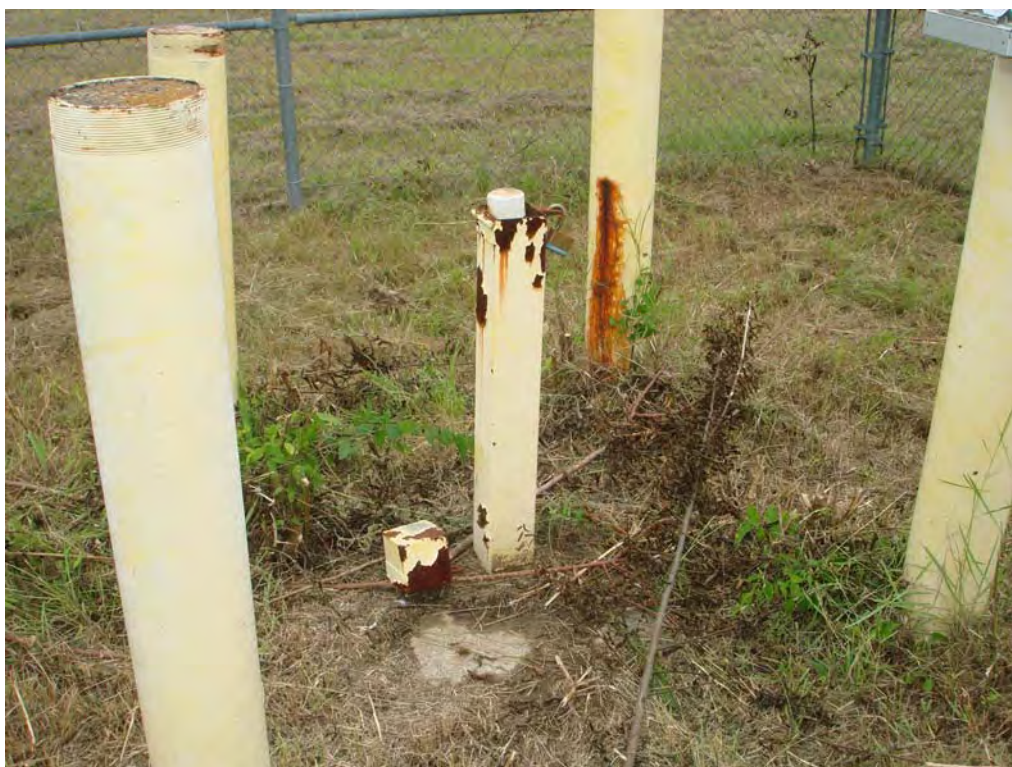
Photograph No. 12 Site: Highlands Acid Pit Superfund Site Description: Monitoring well UA-11 with a broken hinge Date: June 20, 2007
