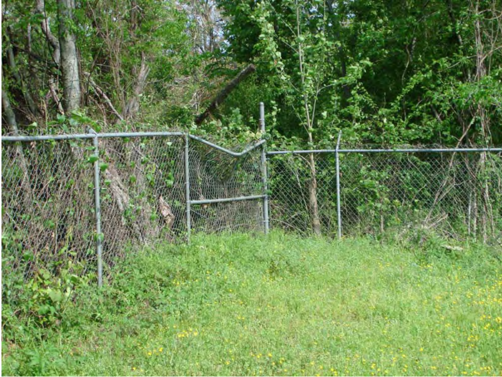
Photograph No. Site: Dutchtown Treatment Plant Superfund Site Description: Damaged perimeter fence northwest corner of site Date: March 29, 2007
