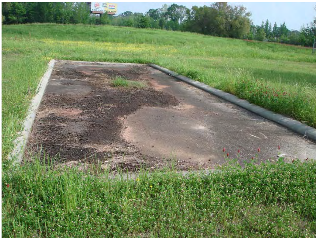
Photograph No. 5 Site: Dutchtown Treatment Plant Superfund Site Description: Onsite concrete pad near center of site Date: March 29, 2007 (note cap elevation in background)
