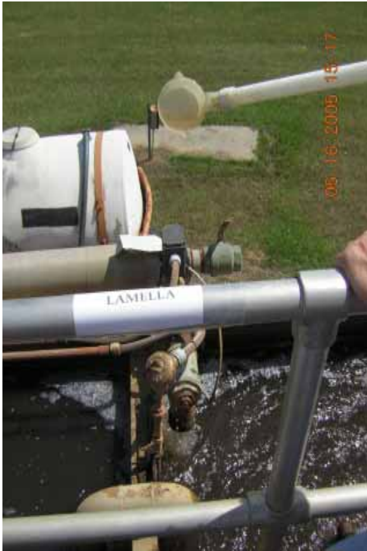
Photo 10: View of water inside the first cell of the bioreactor.
