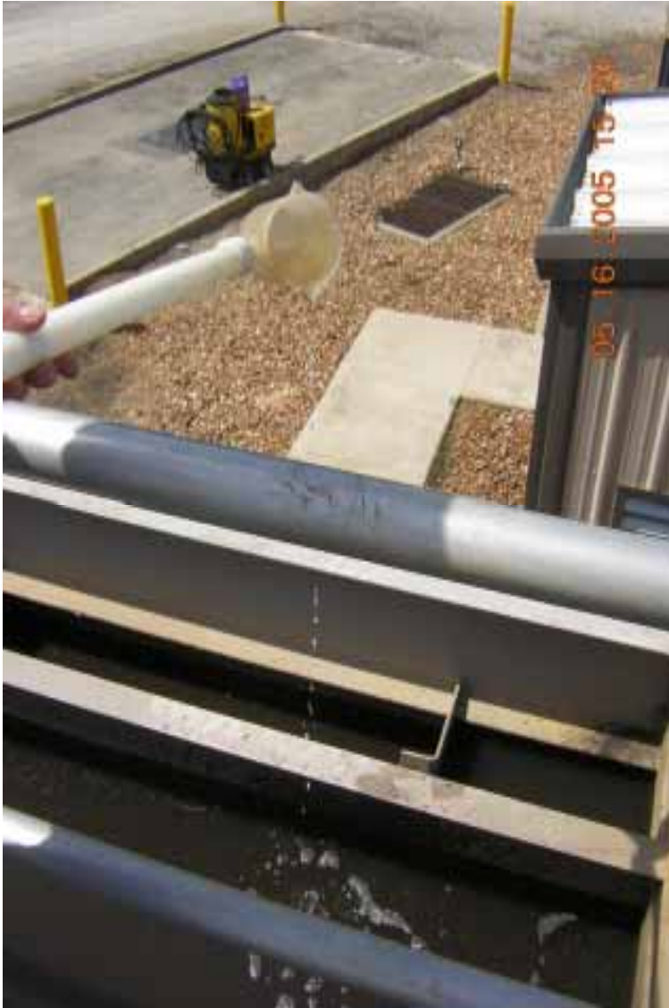
Photo 12: View of water in the last cell of the bioreactor.
