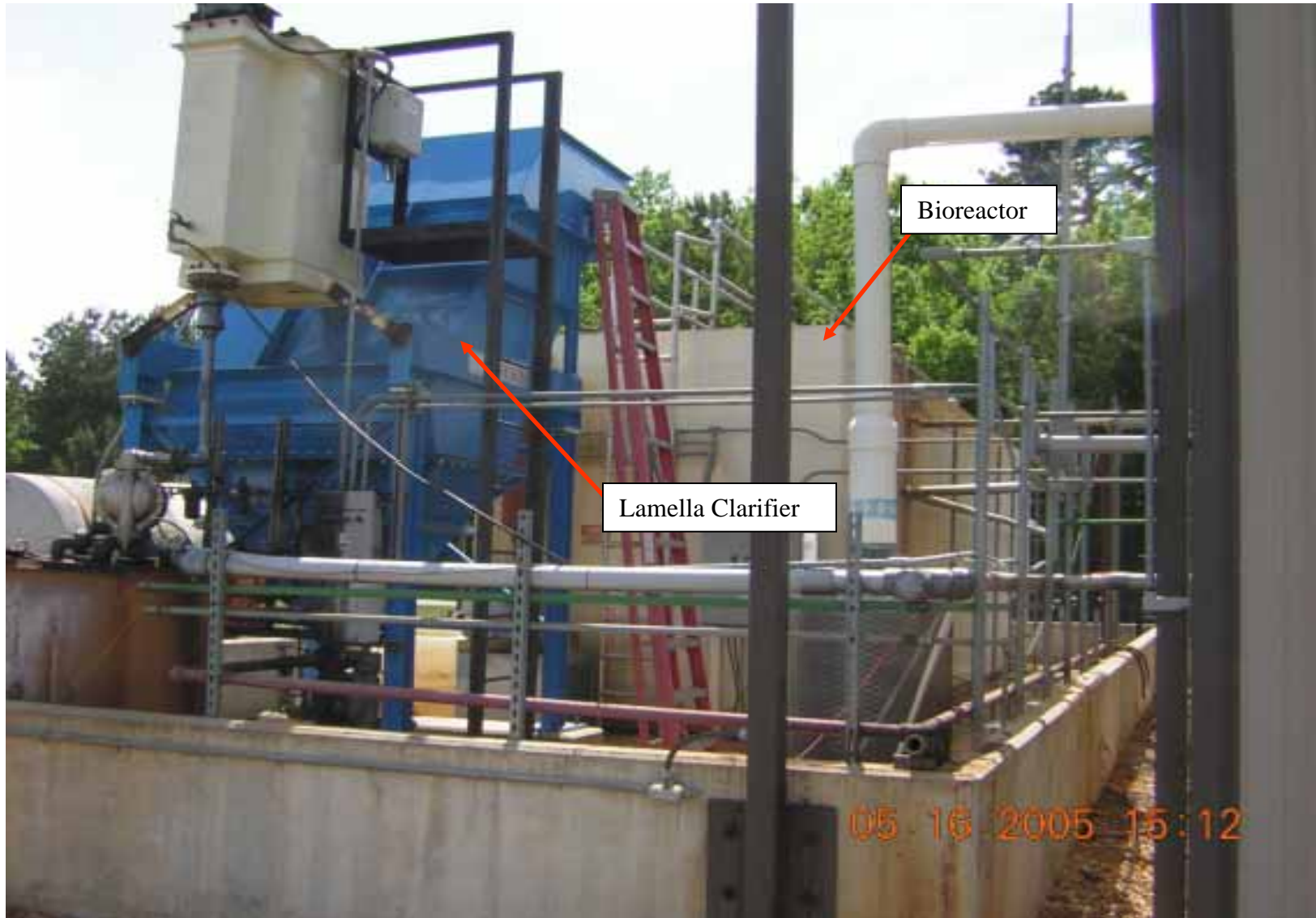
Photo 9: View of the lamella clarifier and bioreactor located outside the PLTS on the south side of the building.
