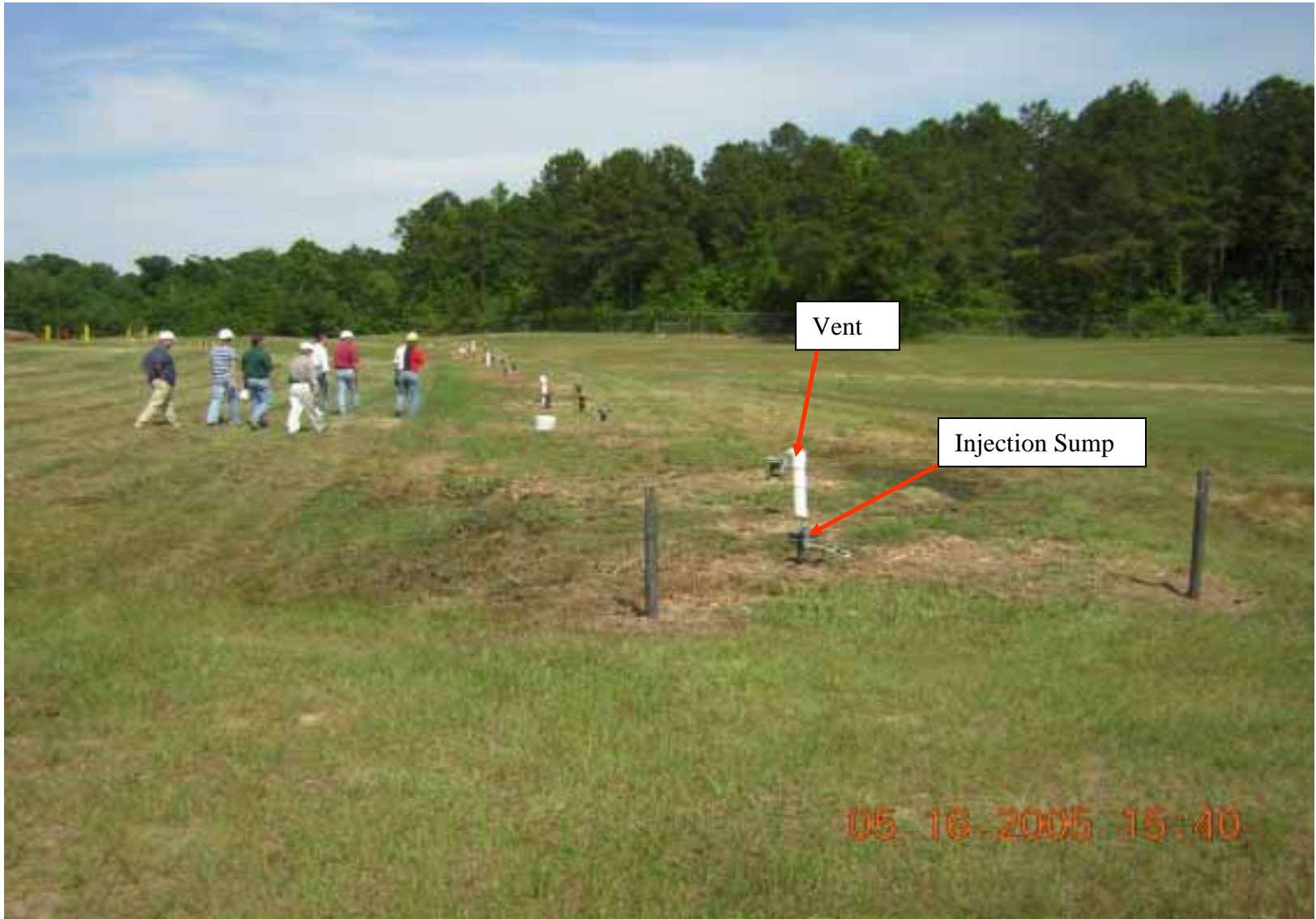
Photo 13: View of the injection trench along the southern portion of the well field.
