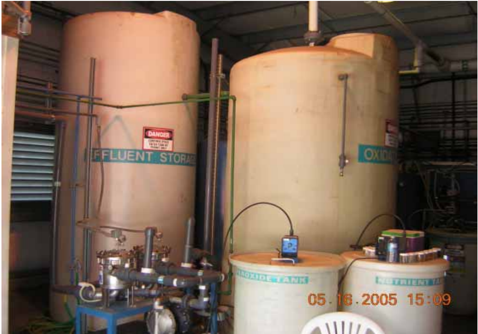
Photo 8: View of the effluent storage tank, and hydrogen peroxide and nutrient amendment tanks inside the PLTS building.
