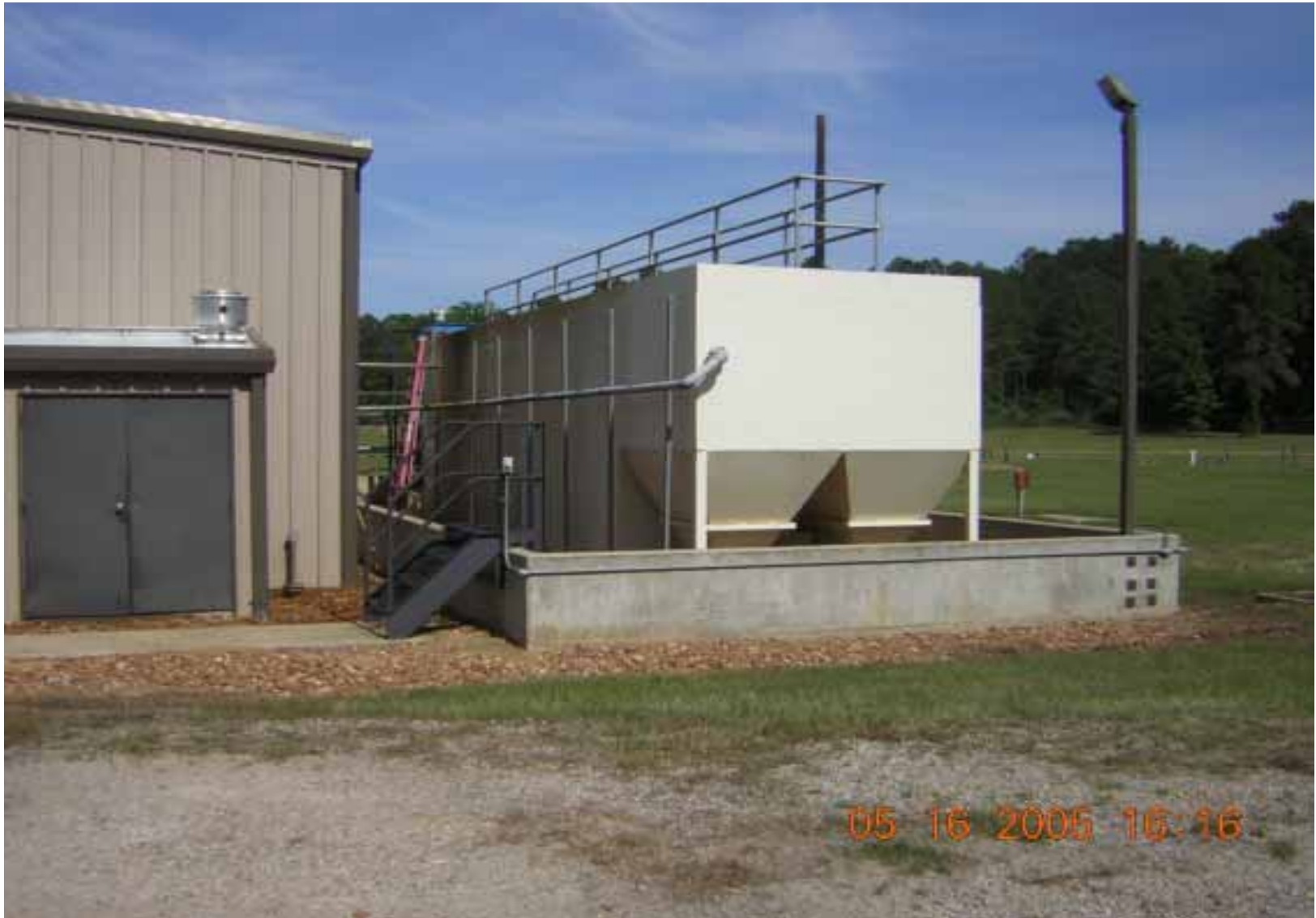
Photo 22: view of the bioreactor facing east.
