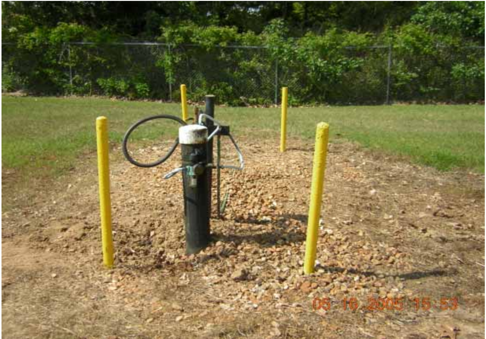
Photo 18: View of a sump in the recovery well.
