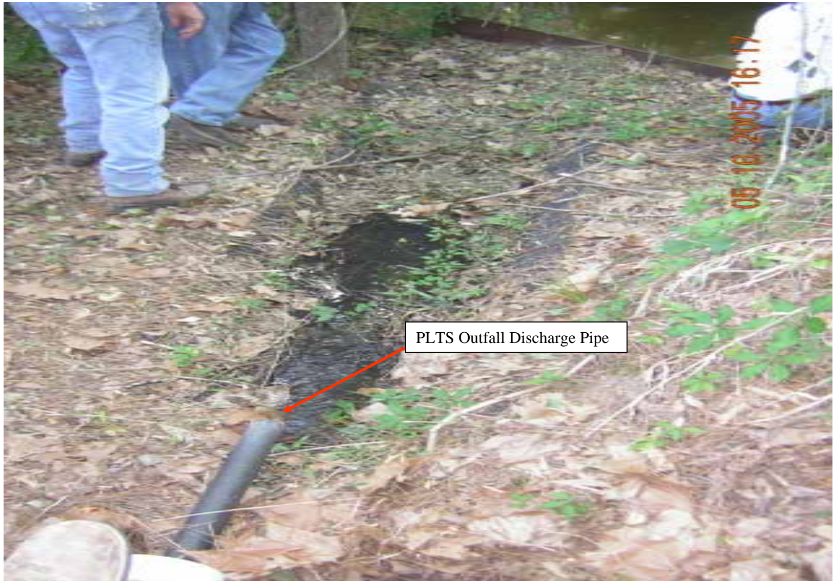
Photo 24: PLTS Outfall discharge pipe.
