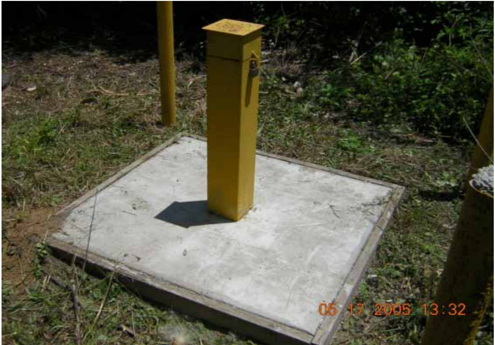
Photo 34: Monitor well SMW-13, located on the north side of Creosote Branch creek.
