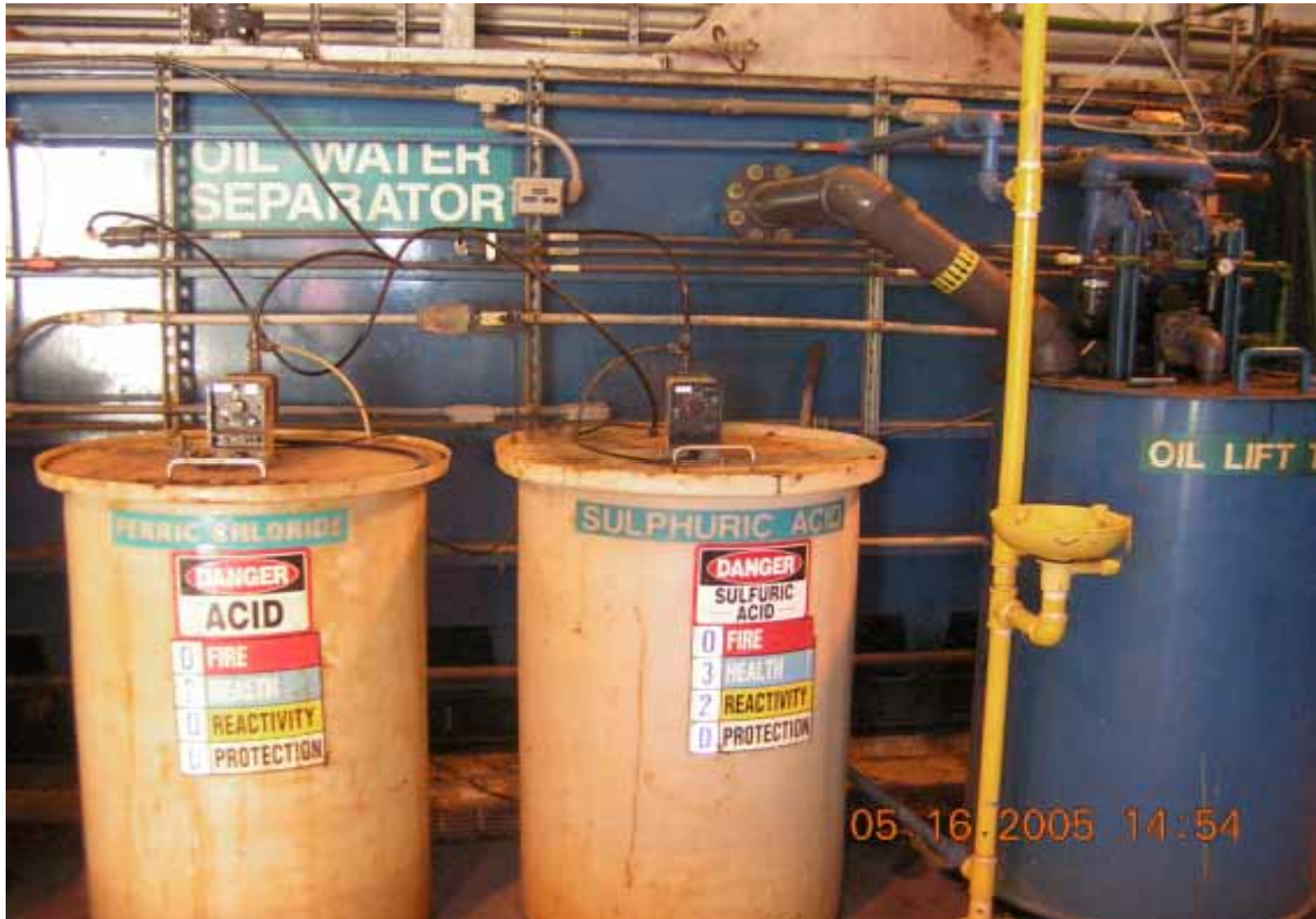
Photo 6: View of the Oil/Water Separator located inside the PLTS.
