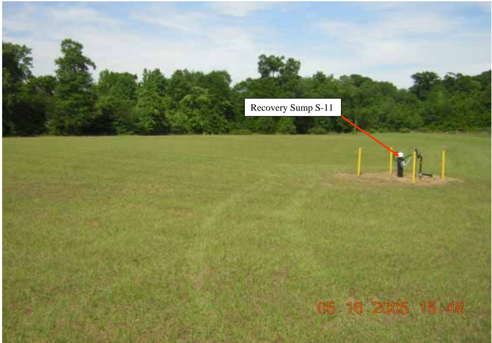
Photo 16: View of the Tar Mat waste burial area facing east. Sump S-11 is at the center-right of the photograph.
