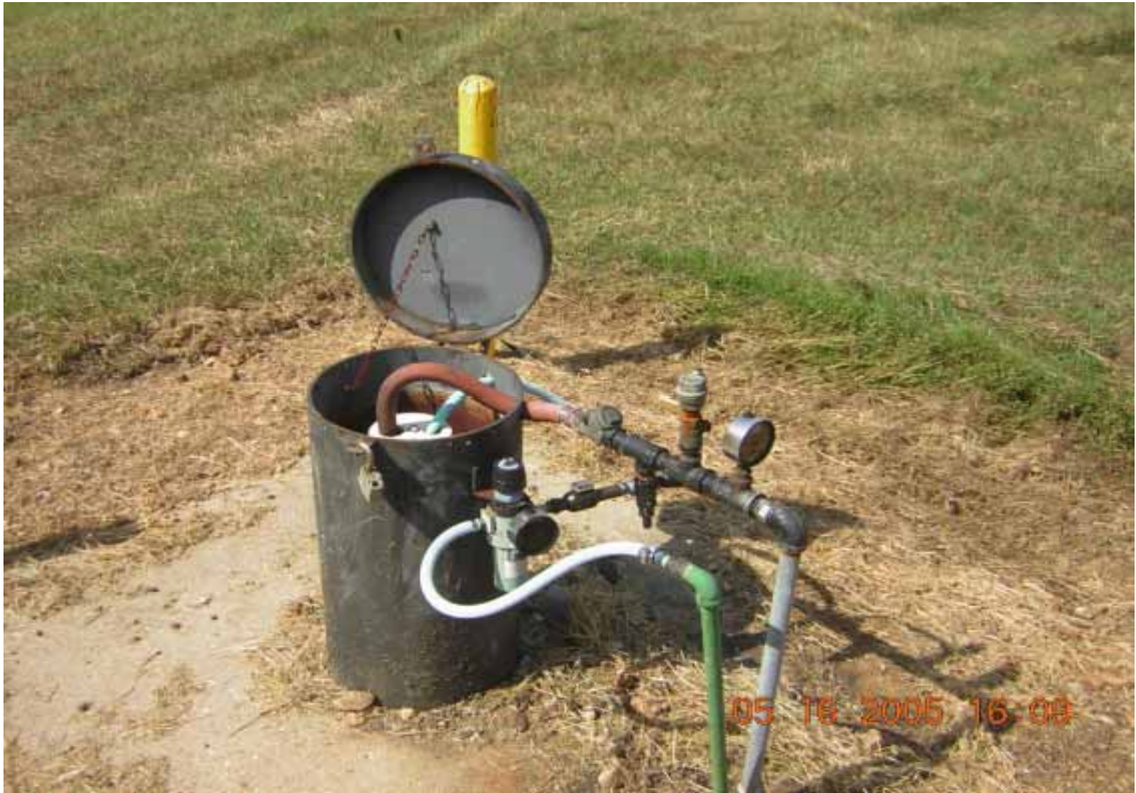
Photo 20: Close-up view of a recovery well.
