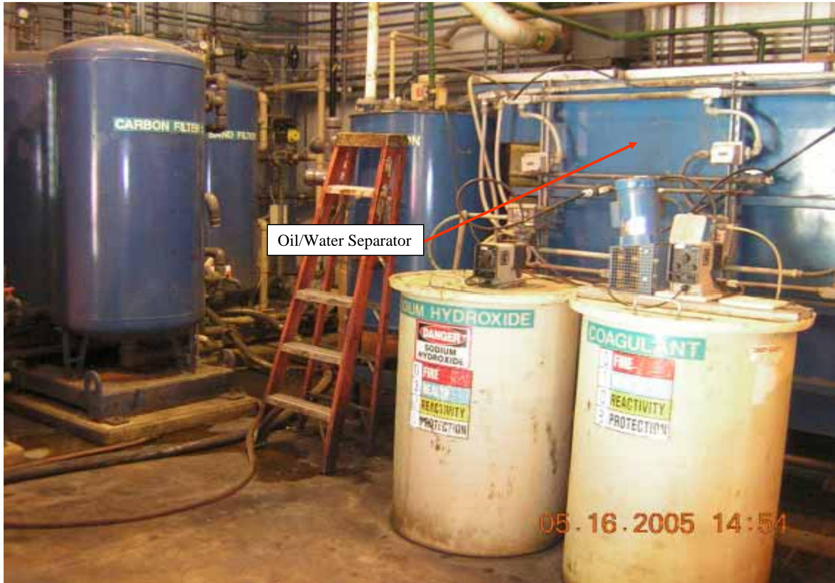
Photo 7: View of the carbon and sand filters inside the PLTS building. The Oil/Water Separator is to the right.
