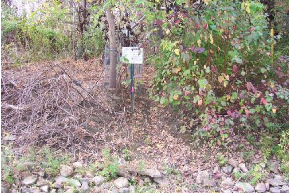
Photo 3 – Downstream Swale: Top-of- bank erosion in Area 1A
