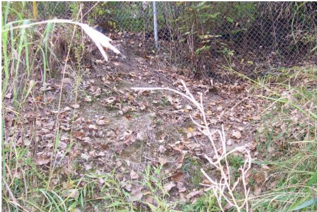
Photo 4 – Upstream Swale: Top-of- bank erosion in Area 1A
