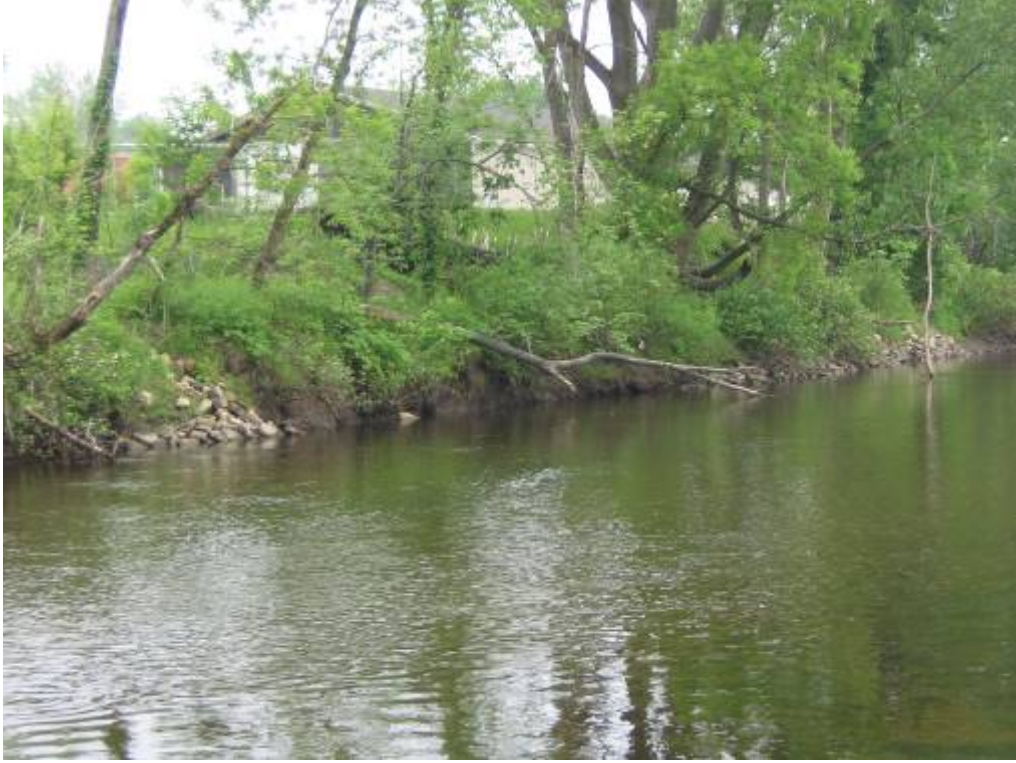
Photo 3 – Area 2: Approximately 100 feet of slight undercut downstream of swale.
