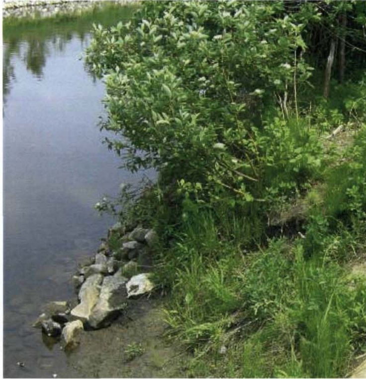
Photo 8 – Area 5: Slight undercut proposed to be armored.
