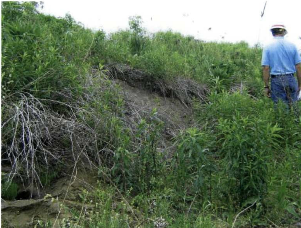
Photo 9 – Area 6: Bank sloughing, no erosion evident.
