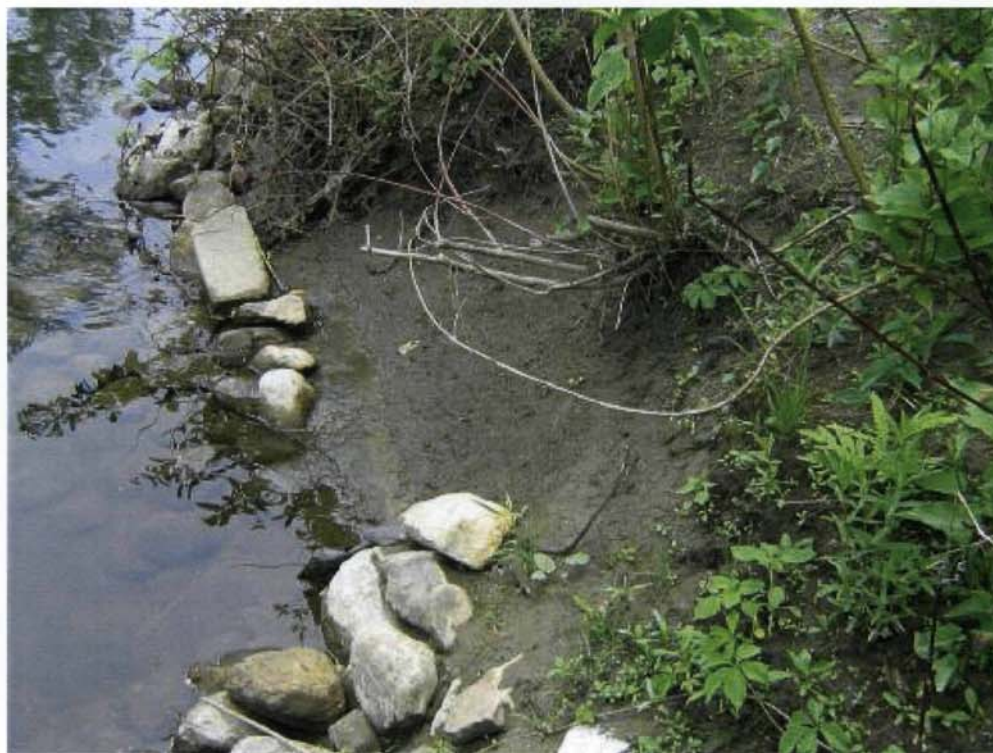
Photo 4 – Area 3: Slight undercut above rip-rap.
