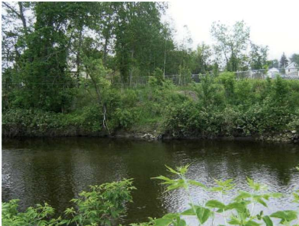
Photo 6 – Area 5: Several small areas undercut above rip-rap.
