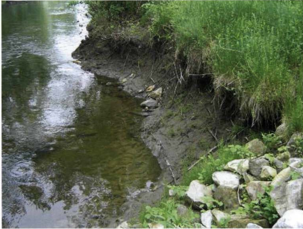
Photo 1 – Area 1: Approximately 25 feet of undercut bank at the end of a section of rip-rap.
