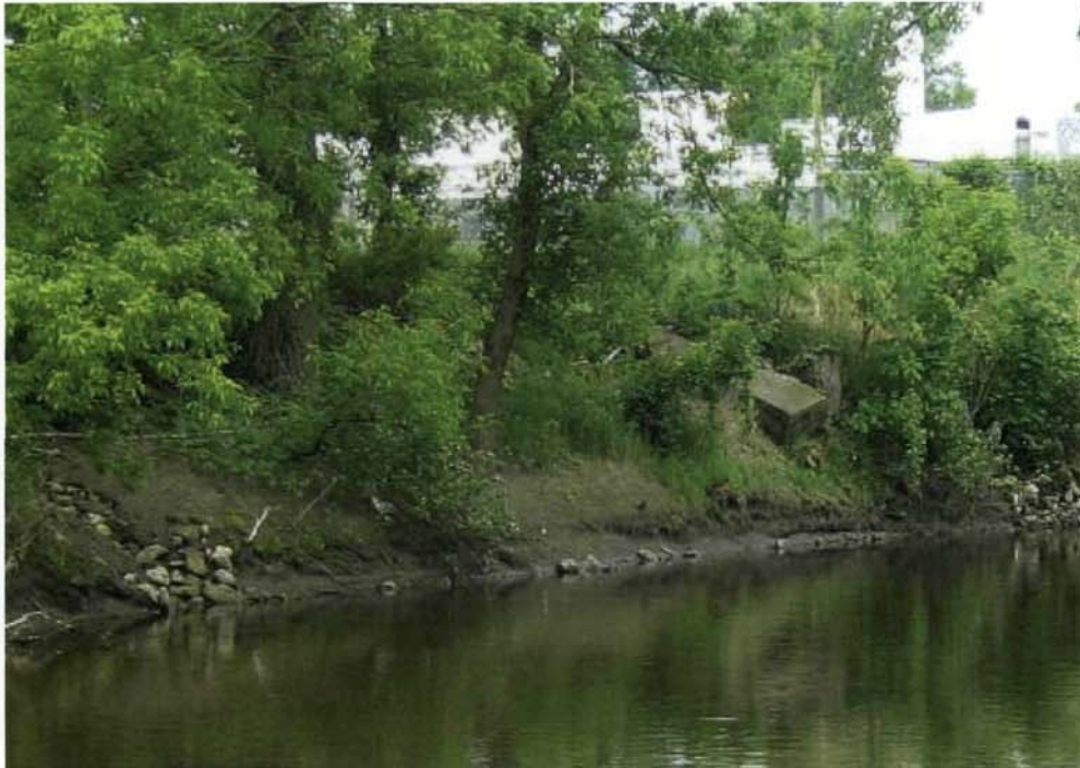
Photo 5 – Area 4: Slight undercut between rip-rap.
