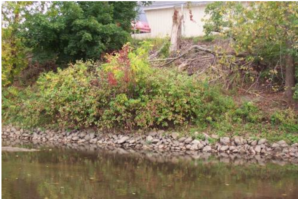
Photo 8 – Area 7: Approximately 30 ft of undercut bank above Riprap
