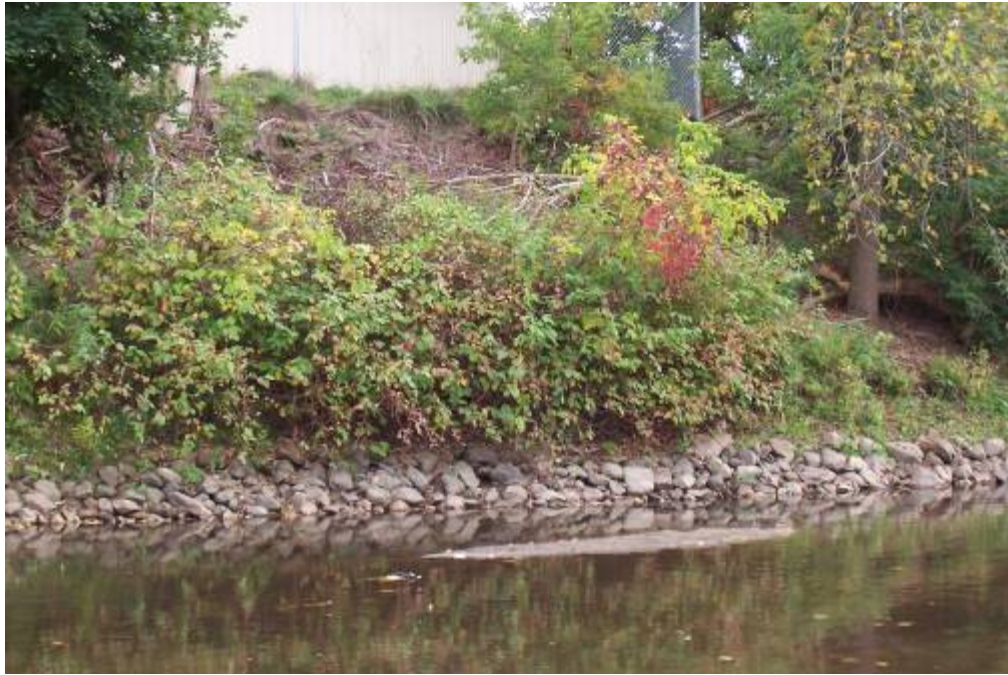
Photo 7 – Area 7: Approximately 30 ft of undercut bank above Riprap
