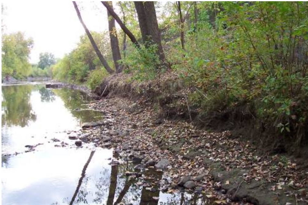
Photo 2 – Area 1A: Approximately 250 ft of undercut bank
