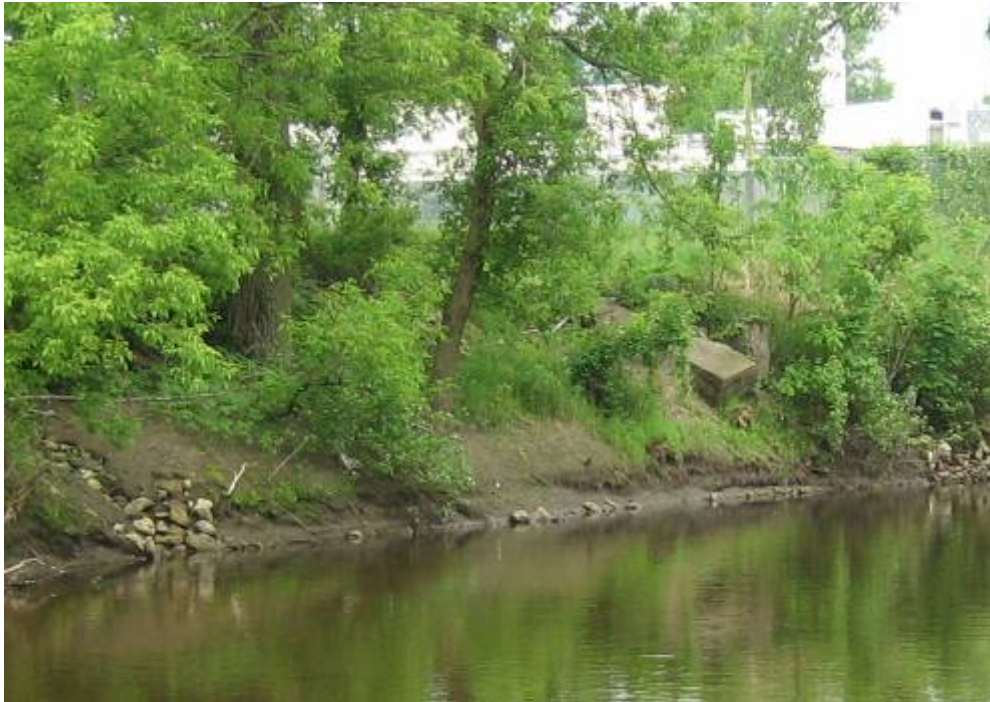
Photo 5 – Area 4: Slight undercut between rip-rap.
