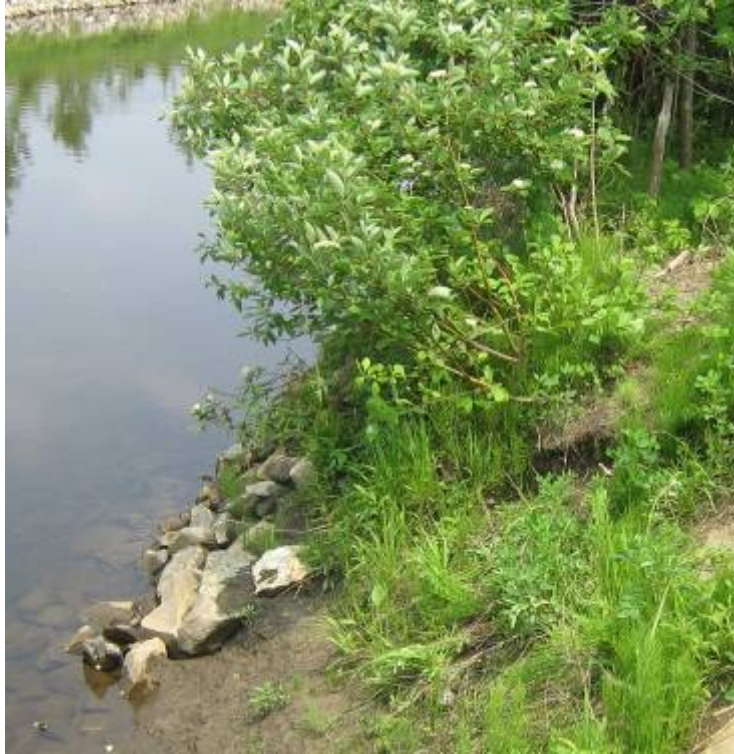
Photo 8 – Area 5: Slight undercut proposed to be armored.
