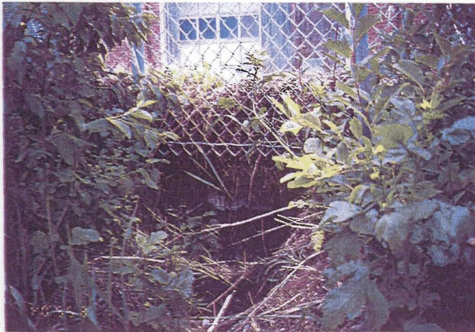
Photo 1 – Area 1: Soil Erosion and Undermining Behind Hay Bale
