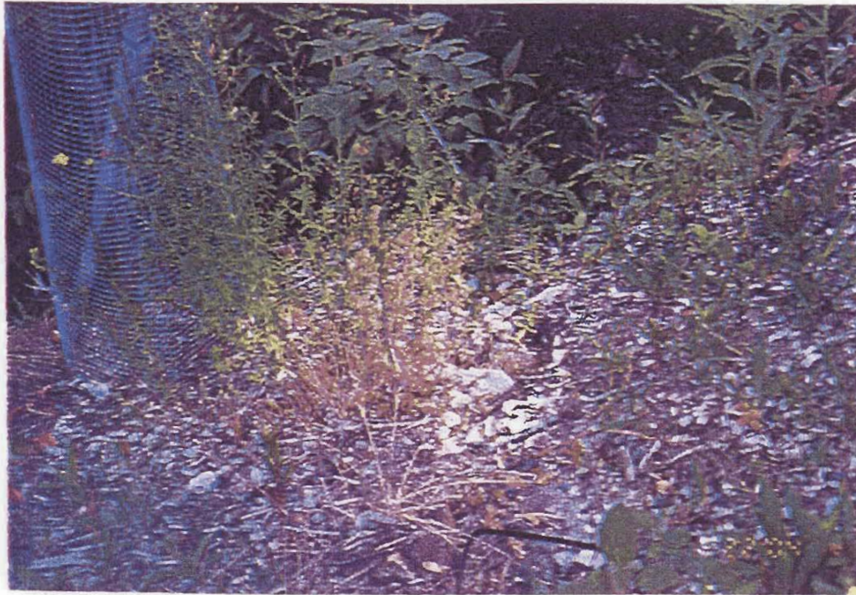
Photo 3 – Area 2: Soil Erosion Near Top-of-Bank
