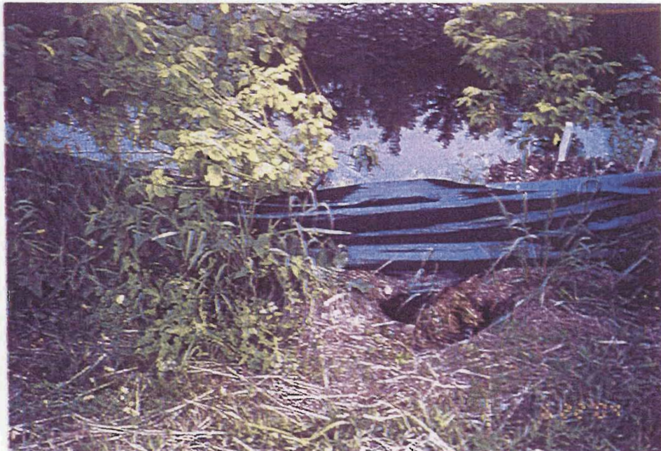
Photo 4 – Area 3: Soil Erosion Near Top-of-Bank
