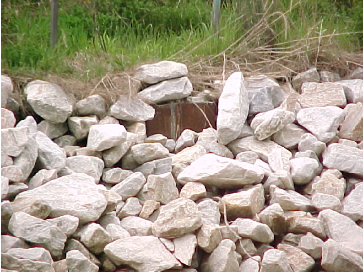
Photo 2 – Area 2: An example of exposed sheeting due to shifted rip rap.
