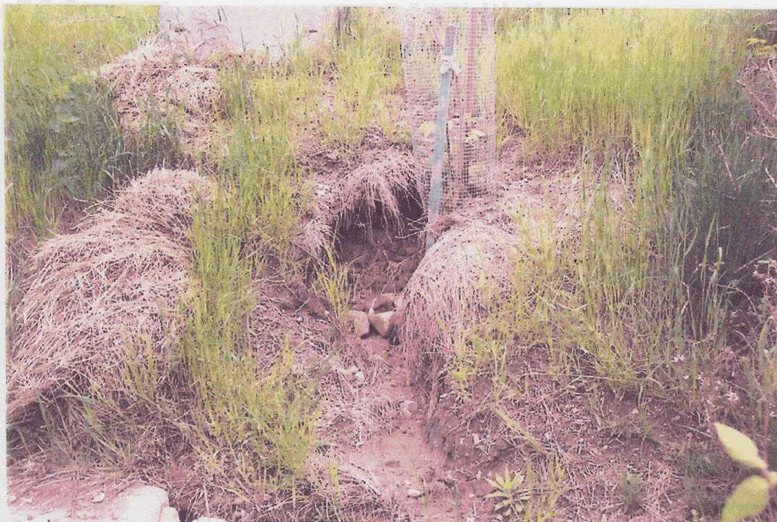
Photograph 5: Spring 2003 Restored Banks Erosion Inspection Area 1 Soil Erosion above Headwall
