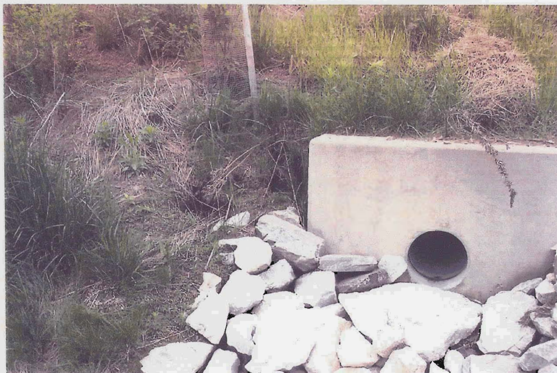
Photograph 6: Spring 2003 Restored Banks Erosion Inspection Area 1 Rip Rap Movement Downstream of Headwall
