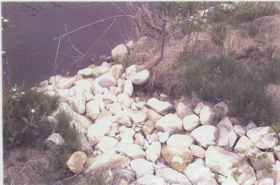
Photograph 8: Spring 2003 Restored Banks Erosion Inspection Rip Rap Movement Swale No. 19 (middle)
