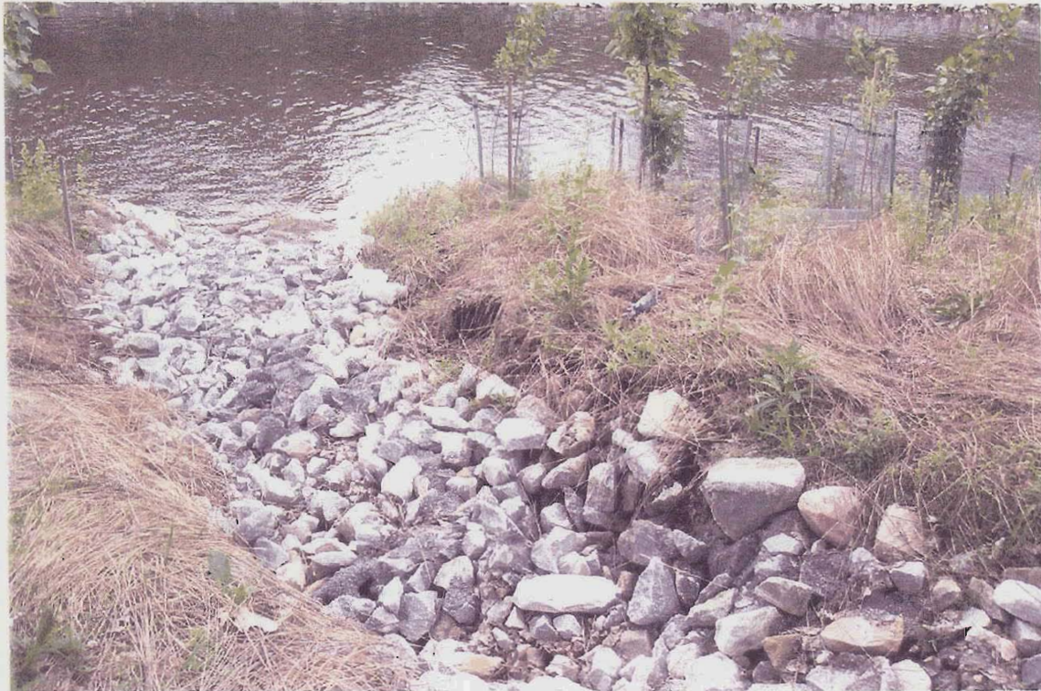
Photograph 7: Spring 2003 Restored Banks Erosion Inspection Settlement/Erosion Swale No. 11
