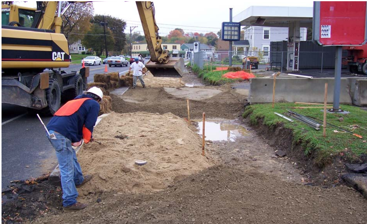
Photo #12: Backfilling and grading of excavation in vicinity of Parcels I8-23-4 and I8-23-5.
