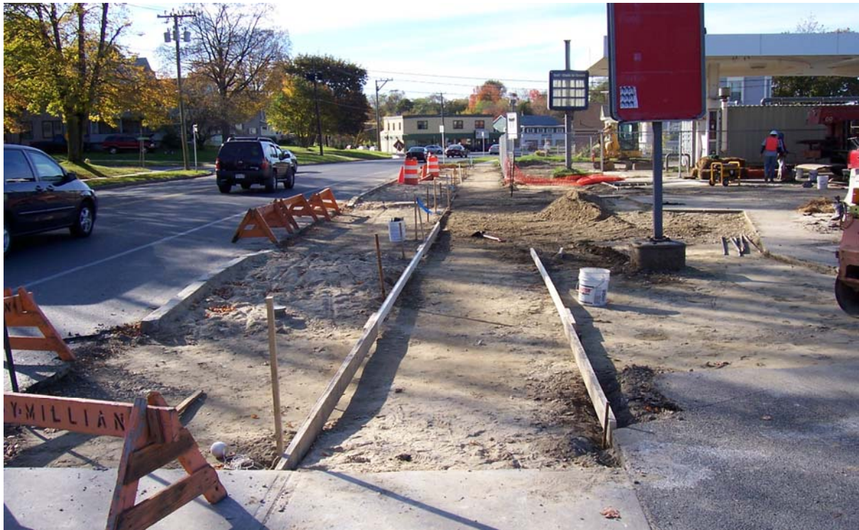
Photo #13: Restoration of concrete/asphalt surfaces in vicinity of Parcels I8-23-4 and I8-23-5.
