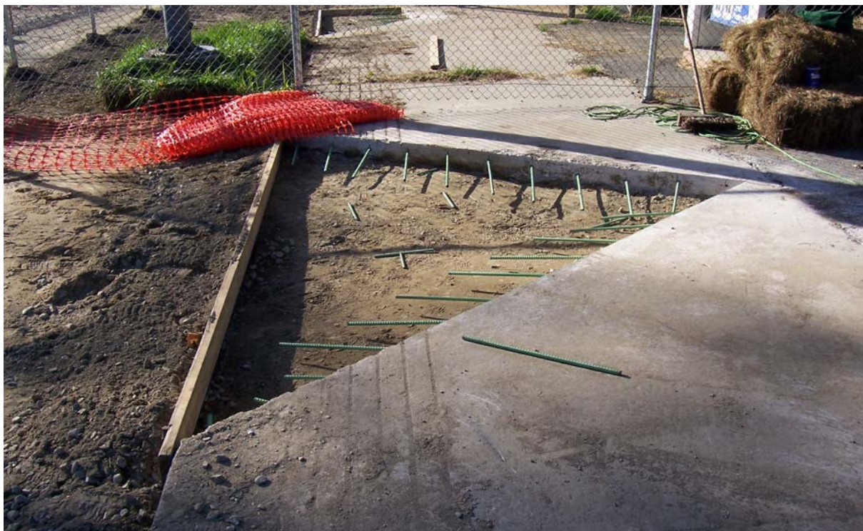
Photo #14: Restoration of concrete surface in vicinity of Parcels I8-23-4 and I8-23-5.
