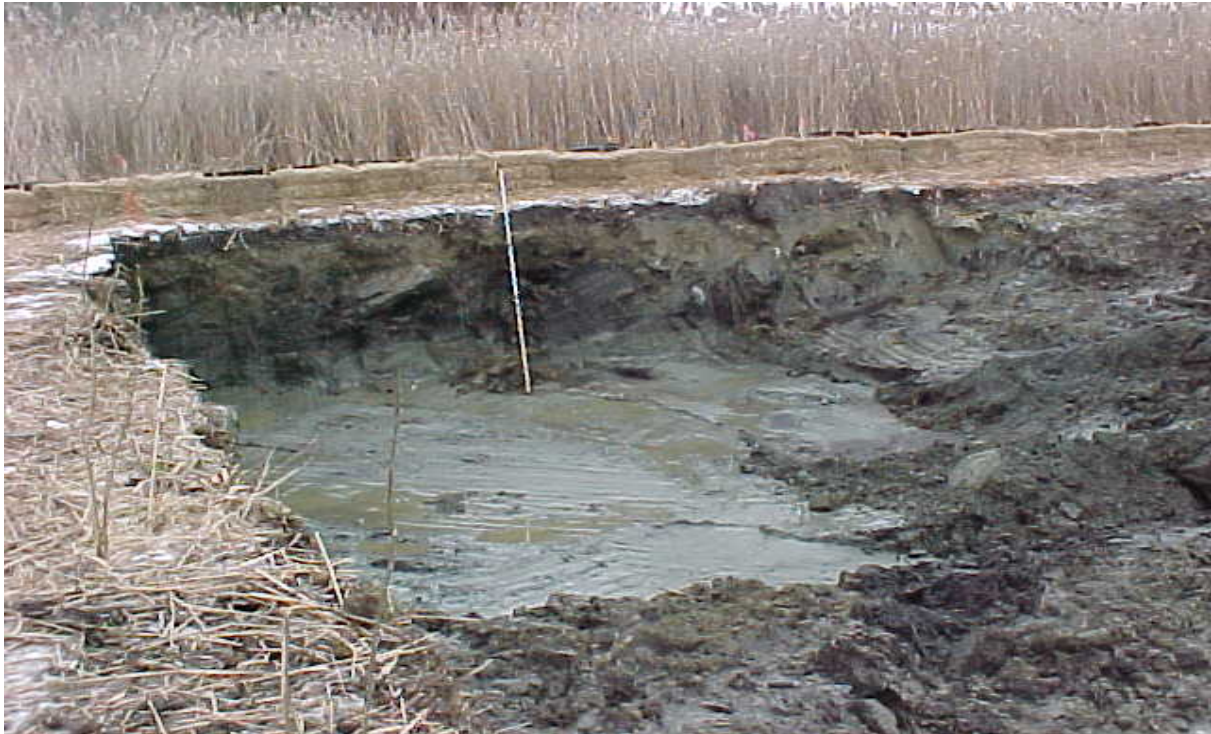
Photo #7: View of completed excavation inside a portion of the removal area.
